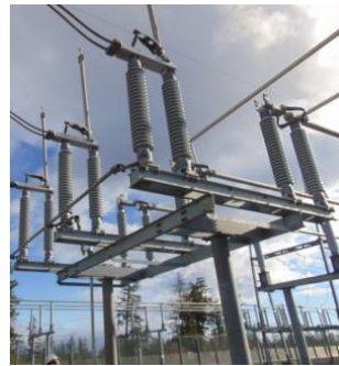
Removed from service
