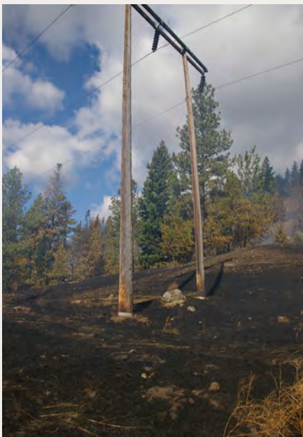
Poles treated with fire protection survive a fire in Falkland in 2011.
