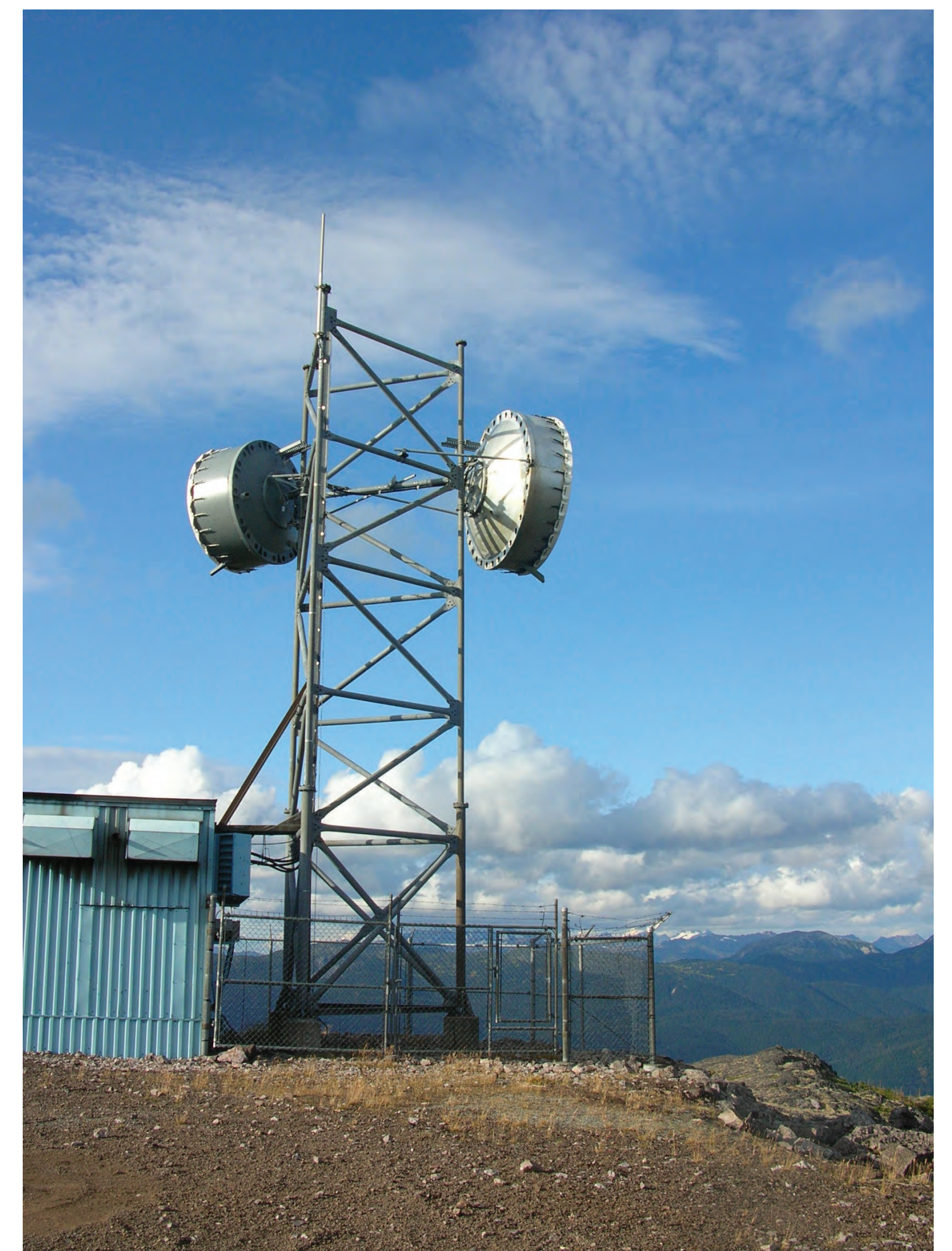
Similar 12m tower with two microwave dishes (1.8 m and 2.4 m). Small building will not be required at this site.
