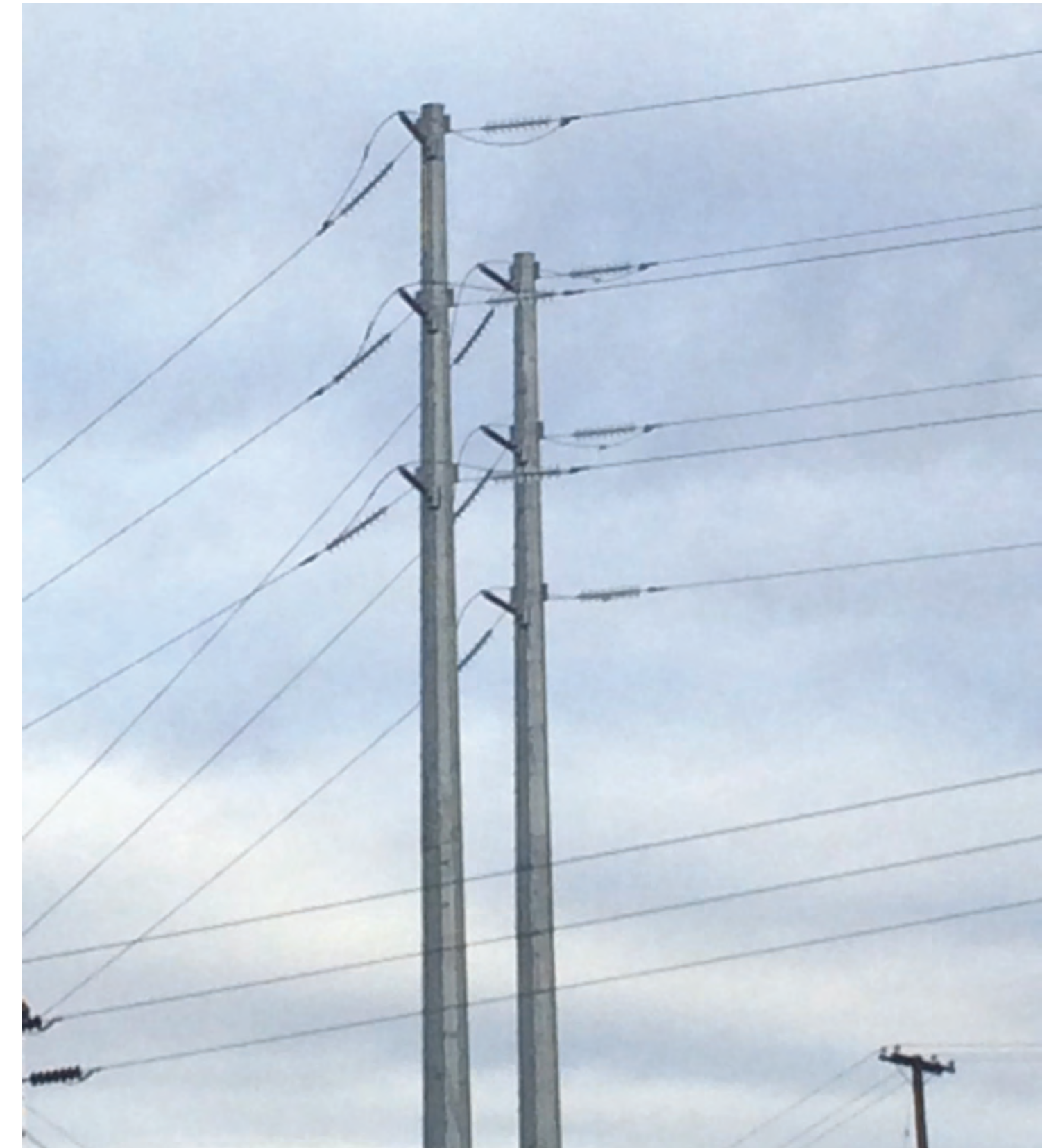
Example of poles (dead ends) to be used next to substation
