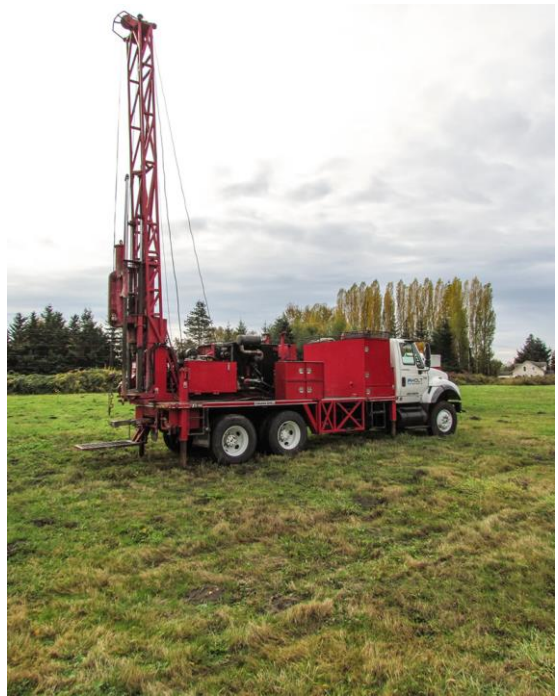
Example of a typical truck-mounted drill rig, similar to what will be used.
