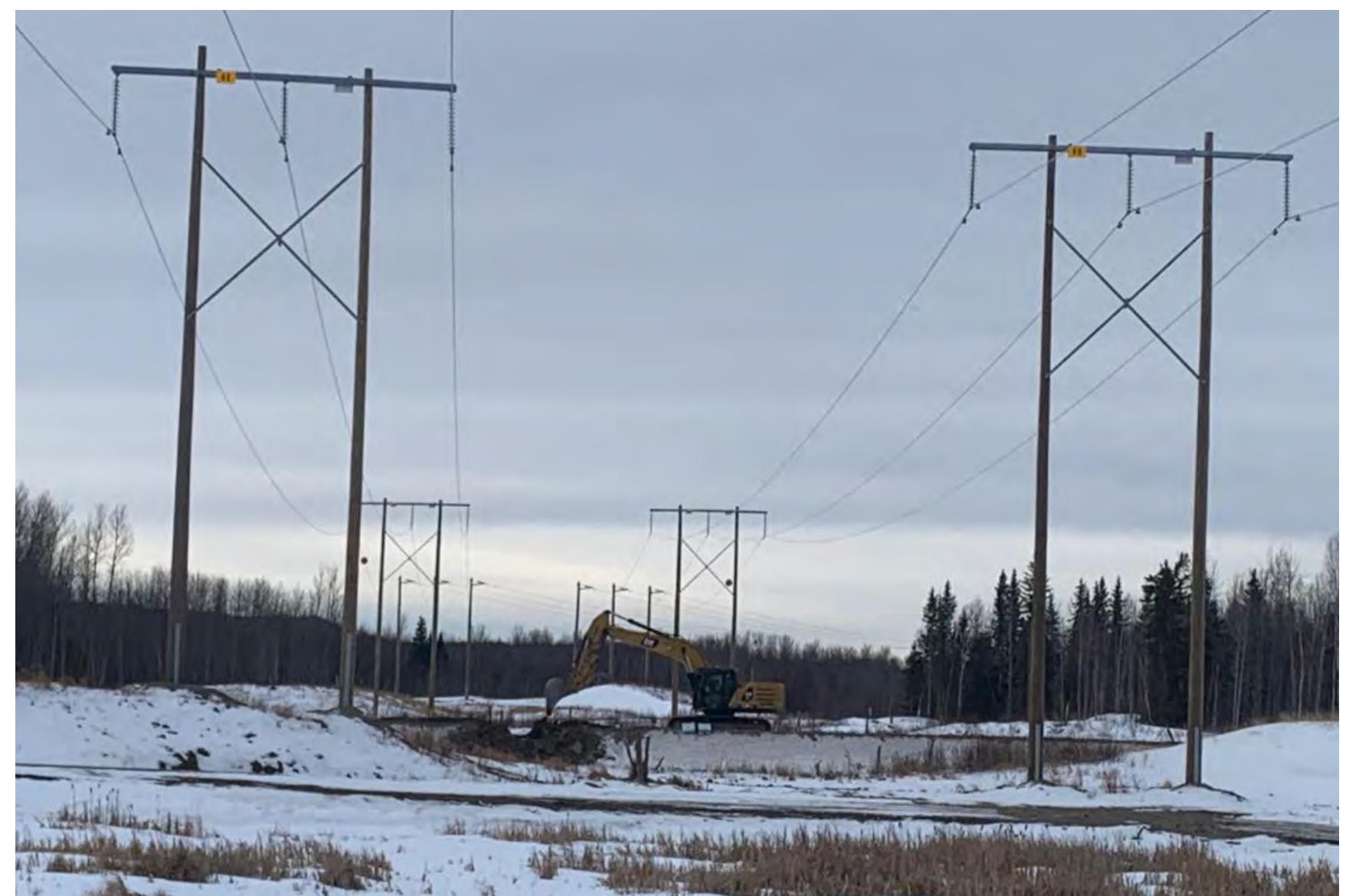
A double circuit span with wooden H frame structures. The line between the new substation and Sparwood is expected to look like this.
