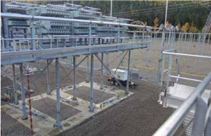
New Seymour Arm series capacitor station.
