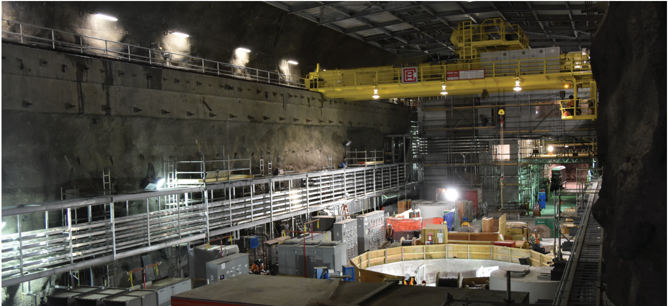
The underground John Hart powerhouse.
