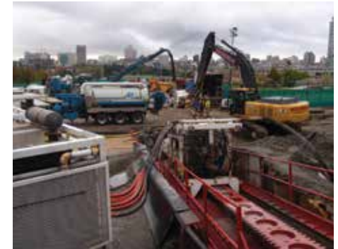
HDD rig and staging area on the Vancouver City Central Transmission (VCCT) Project in David Lam Park, Vancouver
