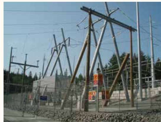
BC Hydro pothead at English Bluff, Tsawwassen. Potheads for this relocation would likely be similar in appearance to this pothead.
