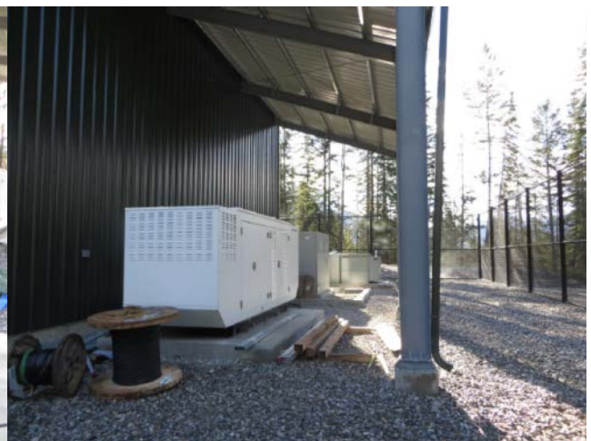
Figure 11 Propane Generator to provide Station backup
