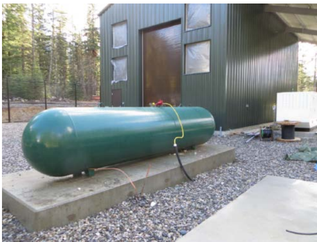
Figure 10 Propane Tank for Station backup Generator
