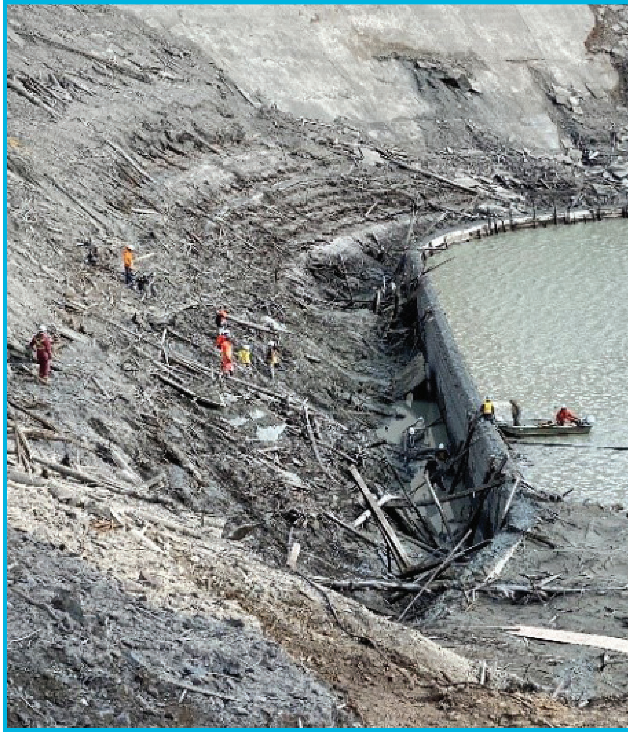
Crews investigating at the toe of the La Joie Dam during the drawdown (April 2022)
