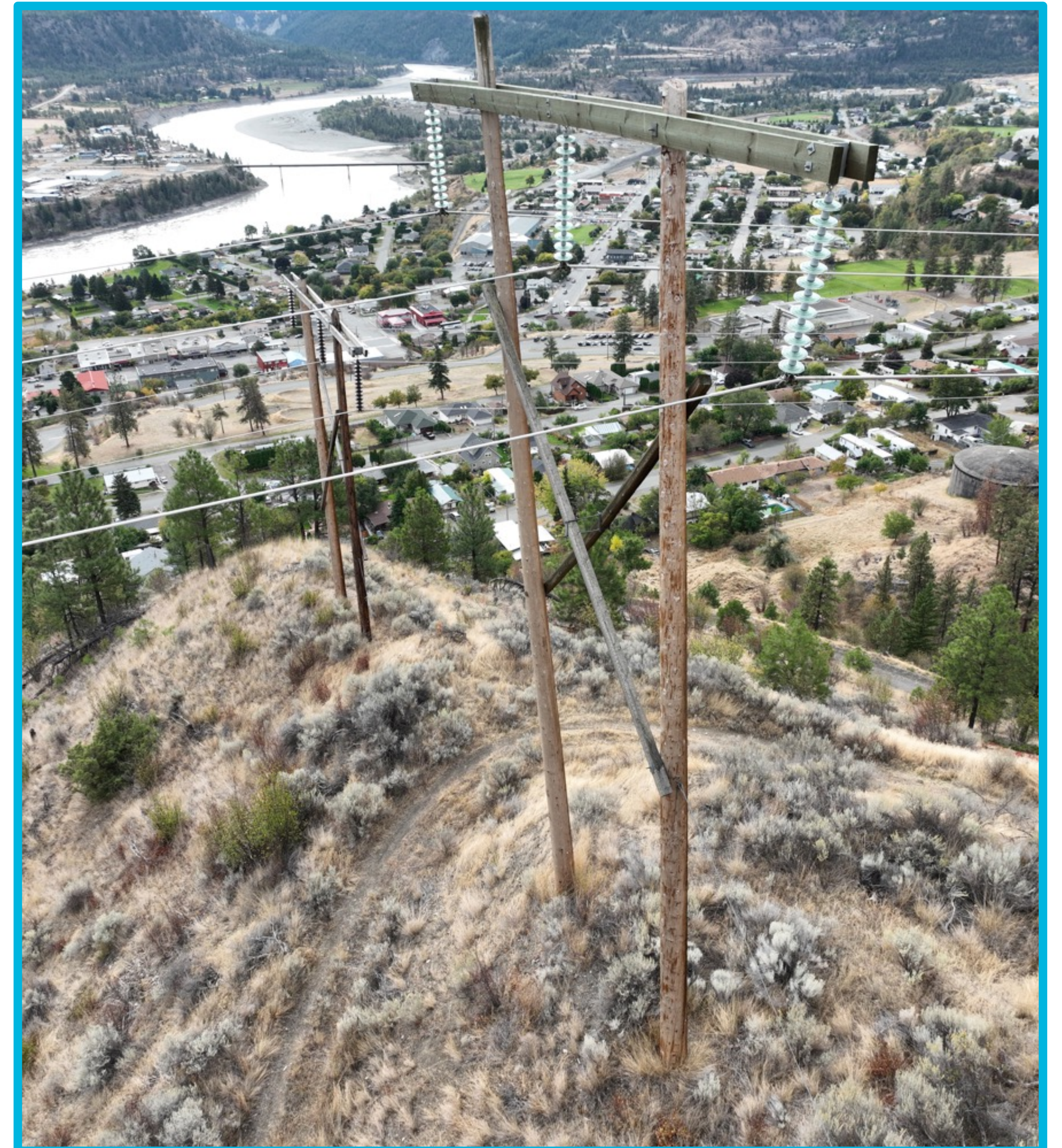
Transmission line 2L90 overlooking Lillooet (2025)
