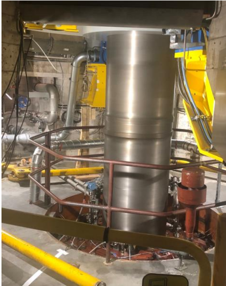
The newly commissioned Unit 7 generator at Bridge 2
