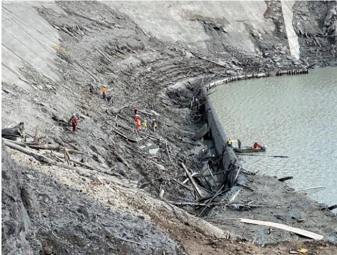
Crews investigating at the toe of LaJoie Dam during the April 2022 drawdown
