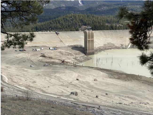
View from Gun Lake Road, looking at the upstream face of LaJoie Dam during the Downton Reservoir drawdown, April 2022
