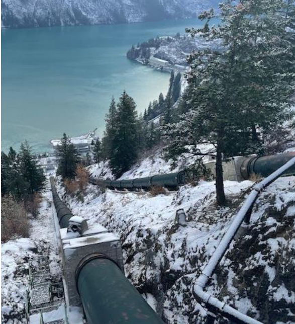
Penstocks running down Mission Mountain to the Bridge 1 powerhouse below with Seton Lake in the background
