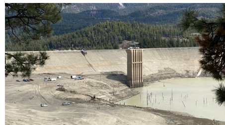
View from Gun Lake Road looking at the upstream face of LaJoie Dam during Downton Reservoir drawdown (April 28, 2022)
