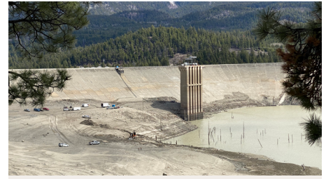
View from Gun Lake Road looking at the upstream face of LaJoie Dam during Downton Reservoir drawdown (April 28, 2022)
