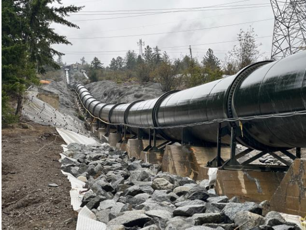
The end of the related GM-0399 penstock foundation refurbishment project that went into service in October 2024.
