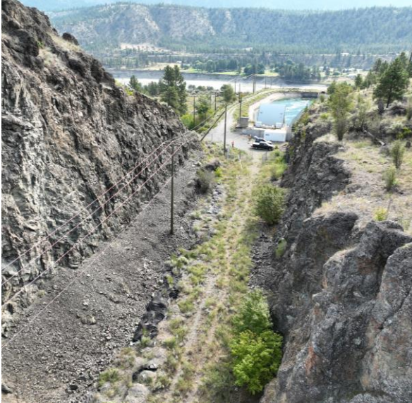
Drone photo of the rock slope along the bypass route with the Seton forebay in the background (July 2023)
