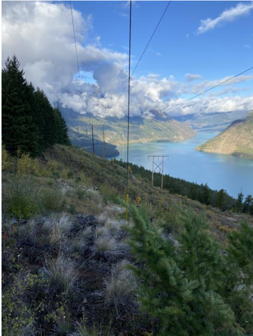
Transmission Line 2L90 running along Seton Ridge.
