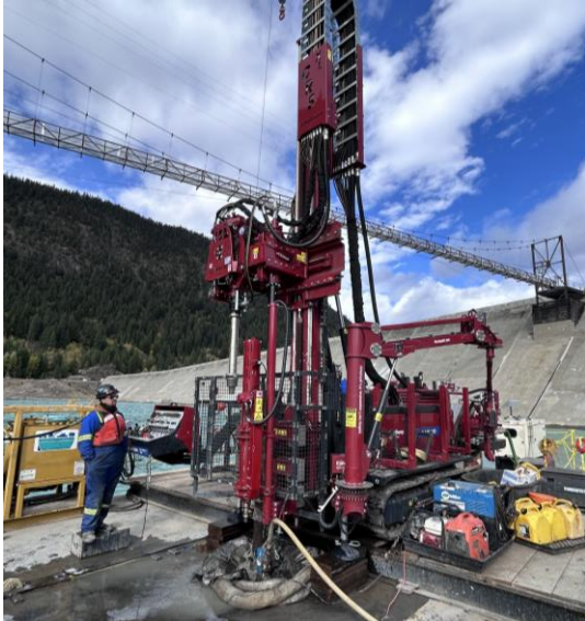
Drillers conducting packer tests on a floating barge near the toe of the dam (October 2024)
