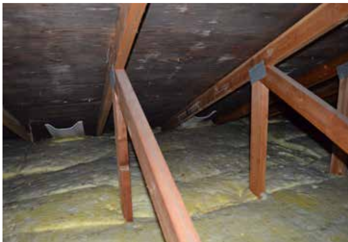
Batt insulation with no gaps
