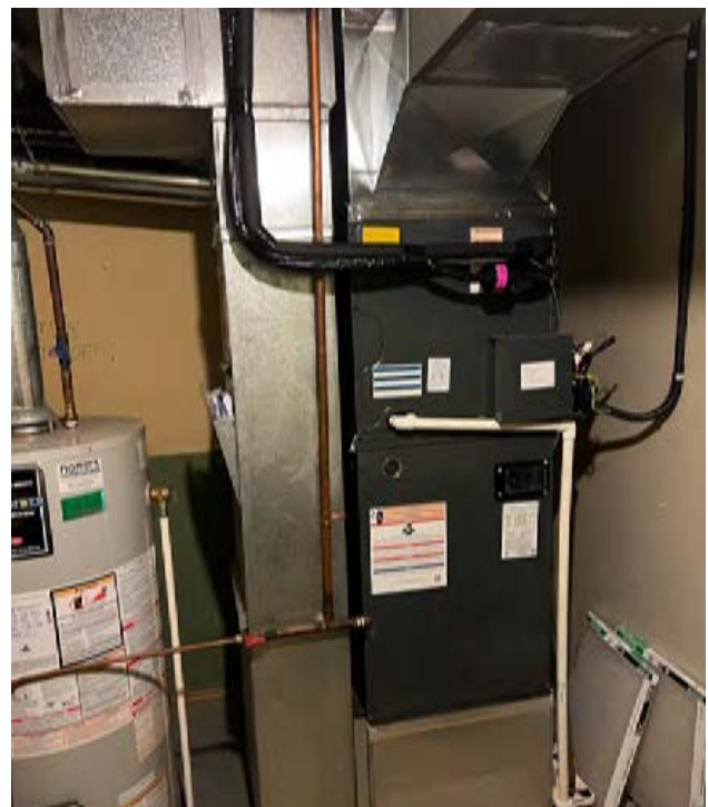
Figure 15 Indoor Unit of a Central Heat Pump
