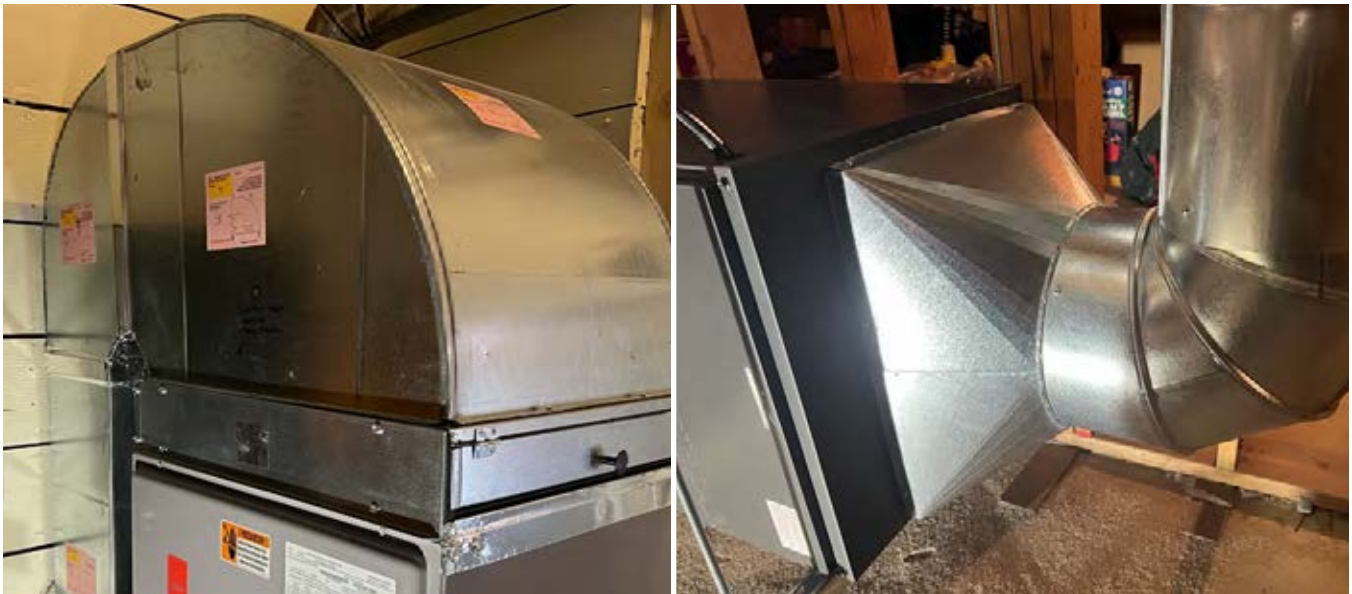
Figure 16 Mechanical Room Duct Transitions that are Properly Sealed and Minimize Static Pressure
