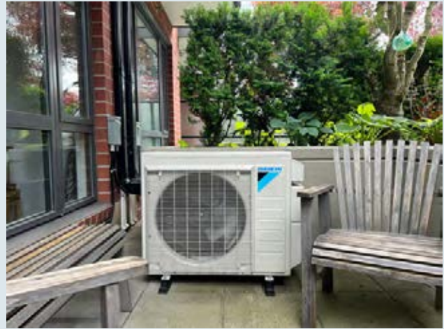
Figure 12 Heat Pump Installed on Level Deck
