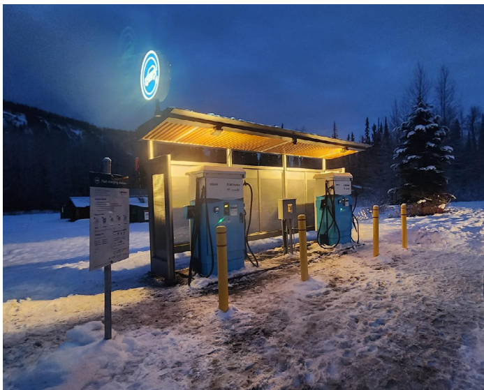
EV charging port weather canopies at Bell 2 Lodge in Northern B.C.
