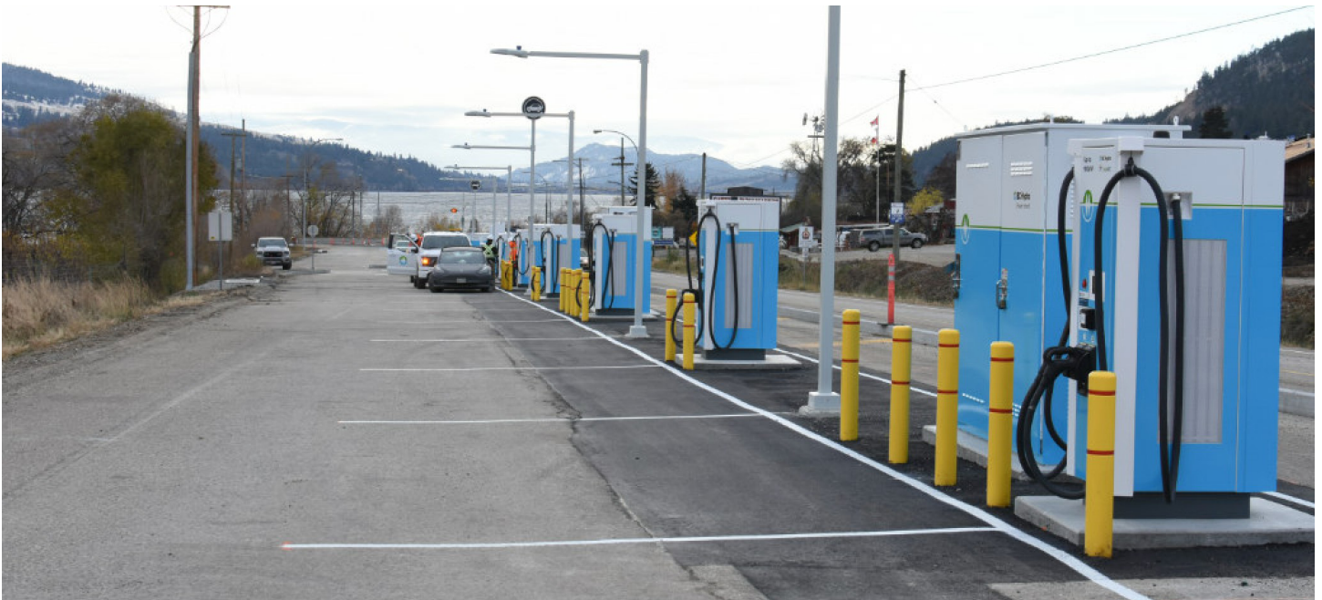
Lake Country charging hub: One of the largest in BC Hydro's network—provides space for up to 22 EVs to charge at the same time and debuted its first 350-kilowatt charger in B.C.
