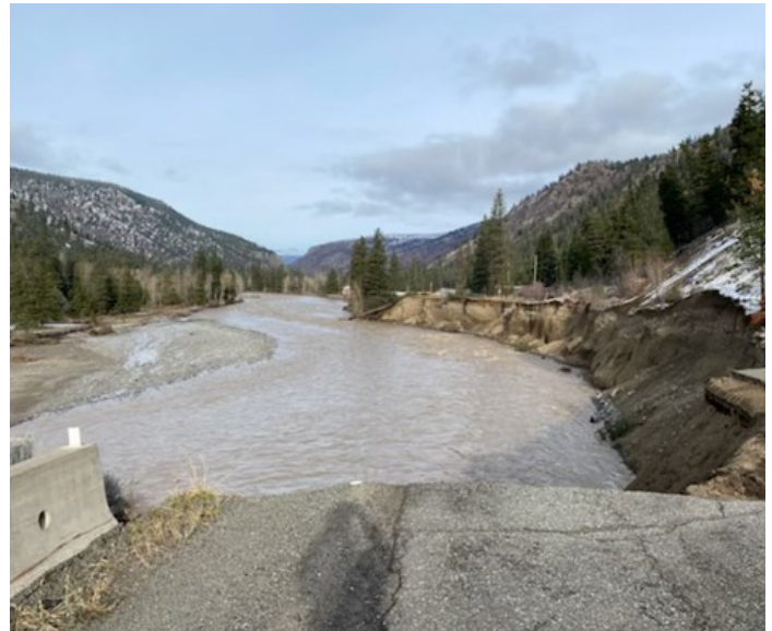
Destruction on the Highway 8 corridor in November 2021
