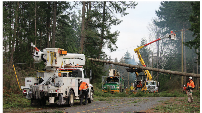
BC Hydro crews hard at work restoring power on Vancouver Island during the 2018 wind storm—the worst storm in BC Hydro's history.
