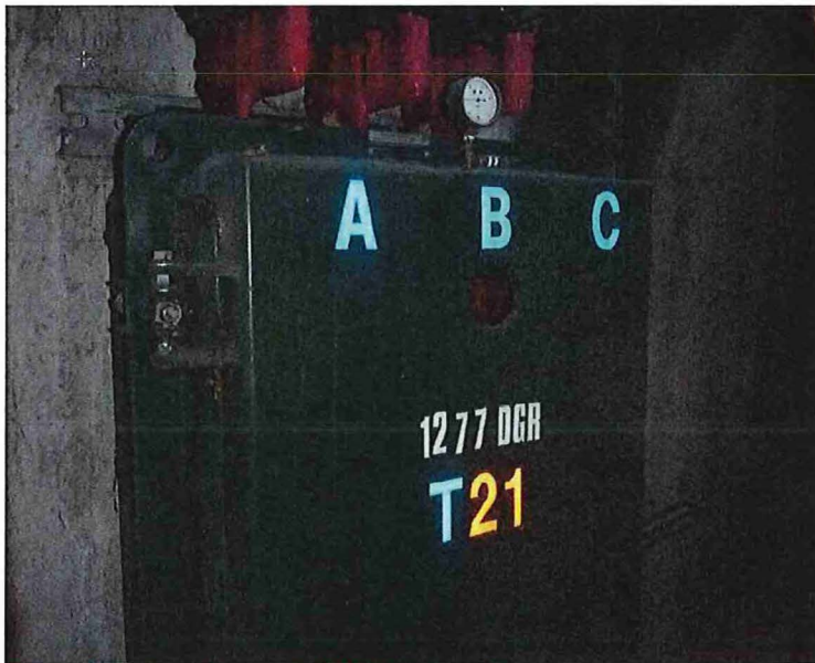
Figure 12 - Spot Network 1500kVA transformer
