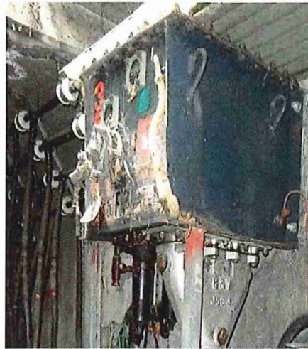
Figure 8 - GRA switch (oil filled)
