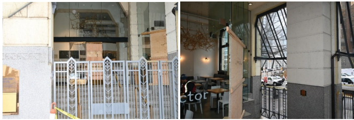
Figure 12: Images showing Tractor restaurant damage.
