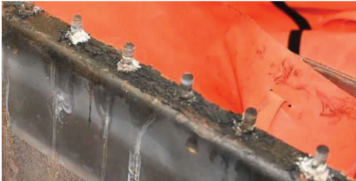
Figure 12. Close up of a region of carbonized and damaged gasket of switch 2018
