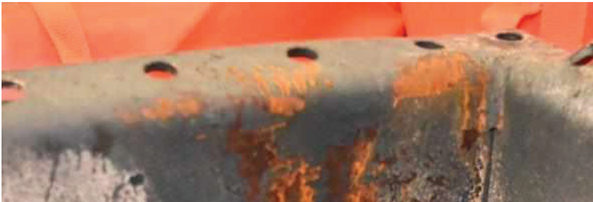
Figure 24. Damage at edge of tank right front
