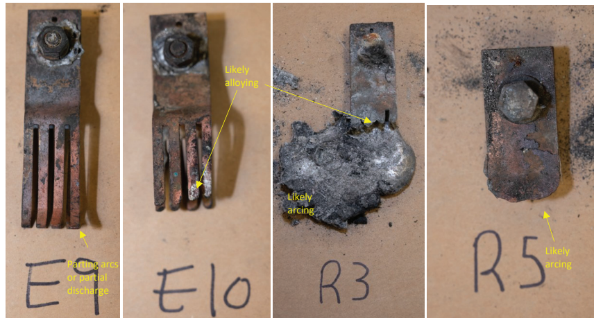
Figure 43: Contact forks found in debris underneath switch (left two), and debris south of switch (right two).
