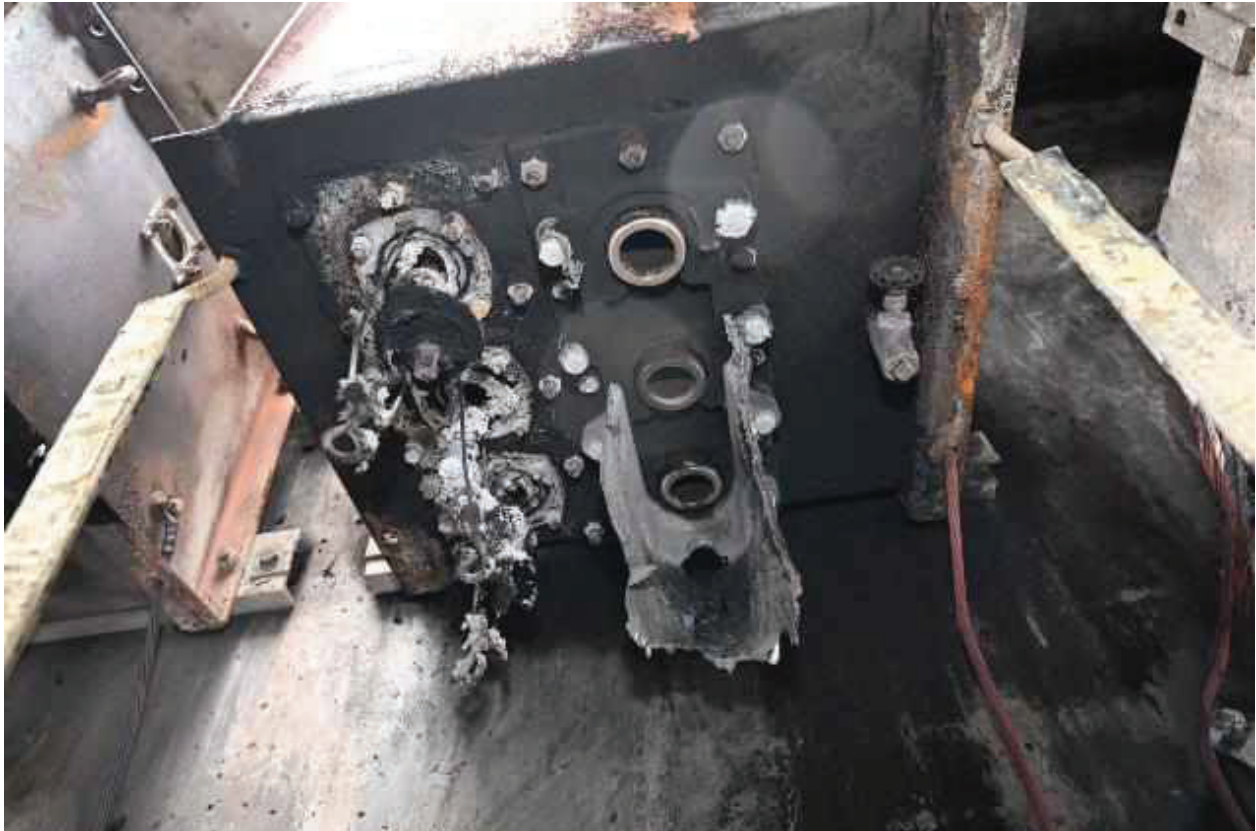
Figure 10. Underside of switch 2018 (in field)
