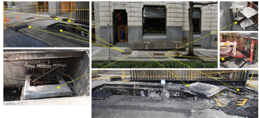
Figure 4: Photo array showing vault debris displacement.
