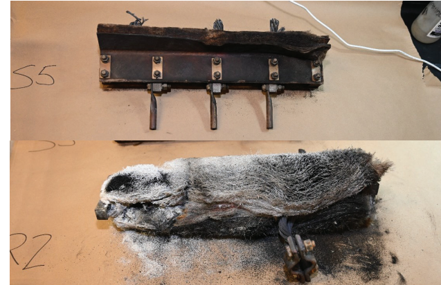
Figure 54: Insulation for Switch Hinge Pins (a) Switch 2018 (Sample S5); (b) Switch 2019 (Sample R2).
