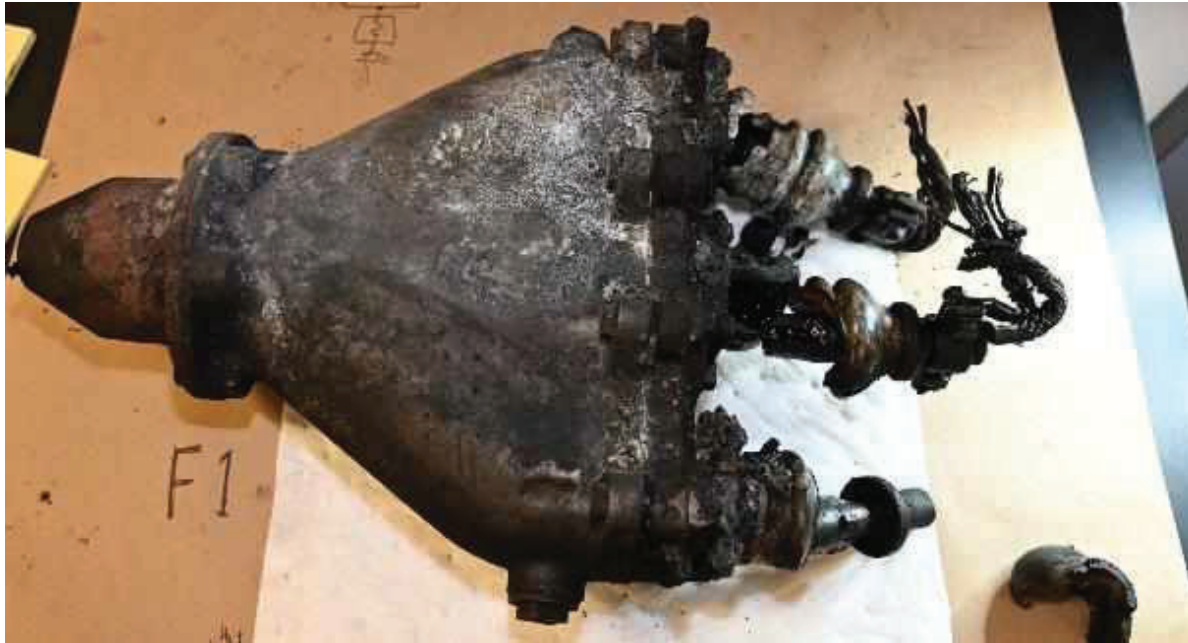
Figure 7. PILC termination from switch 2019
