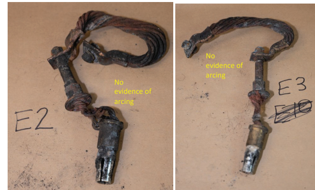
Figure 44: Elbow connector cables found in debris immediately below SW2019.
