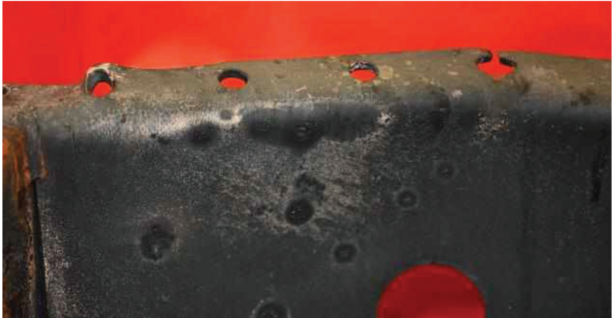
Figure 3. Close up of bolt holes on front right of switch 2019 (view from inside of tank)
