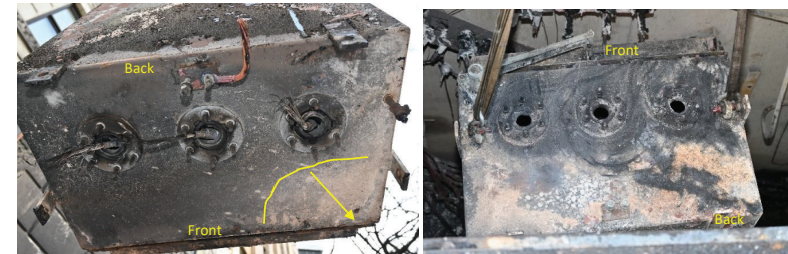
Figure 26: Bottom of CLF cabinet showing broken cables (left); top of CLF cabinet (right).
