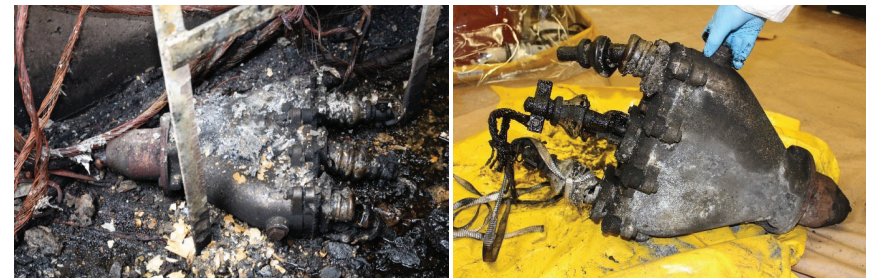
Figure 40: SW2019 PILC Connector and Termination as found (left); in laboratory (right).
