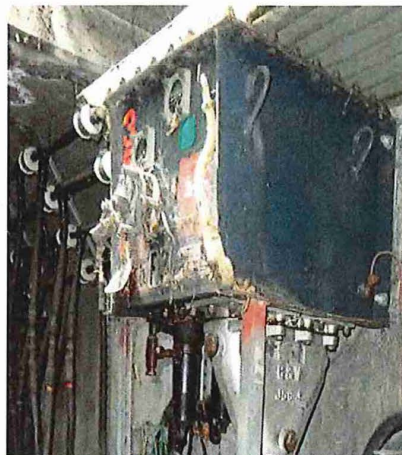
Figure 8 - GRA switch (oil filled)
