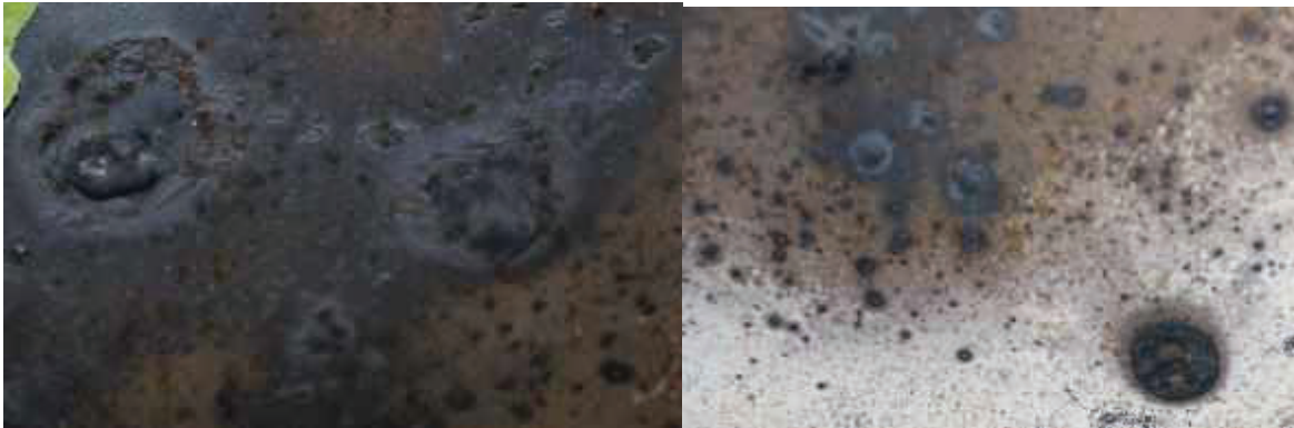
Figure 13. Selected photos of metallic-like splatter on the tank walls of switch 2019
