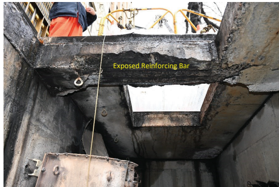
Figure 16: Vault structural damage.
