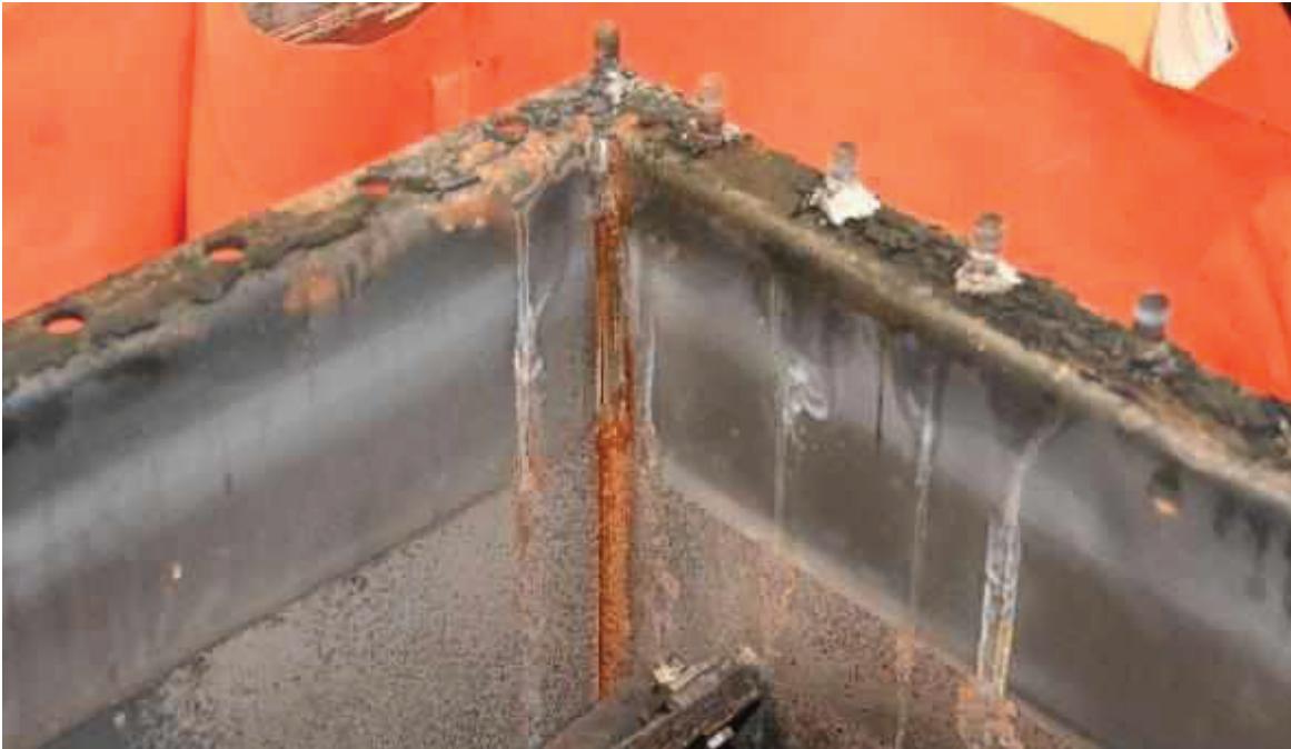
Figure 9. Close up of orange-brown residue on walls of switch 2018
