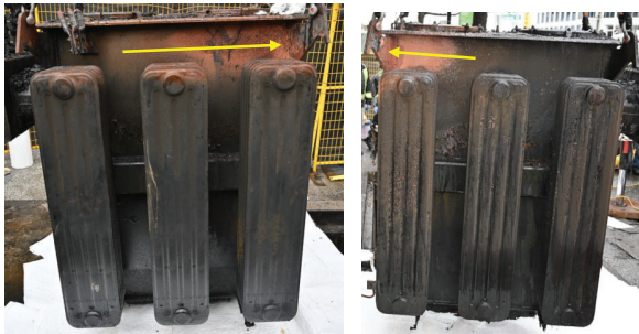
Figure 21: Sides of transformer (a) Left - east side (b) Right - west side.
