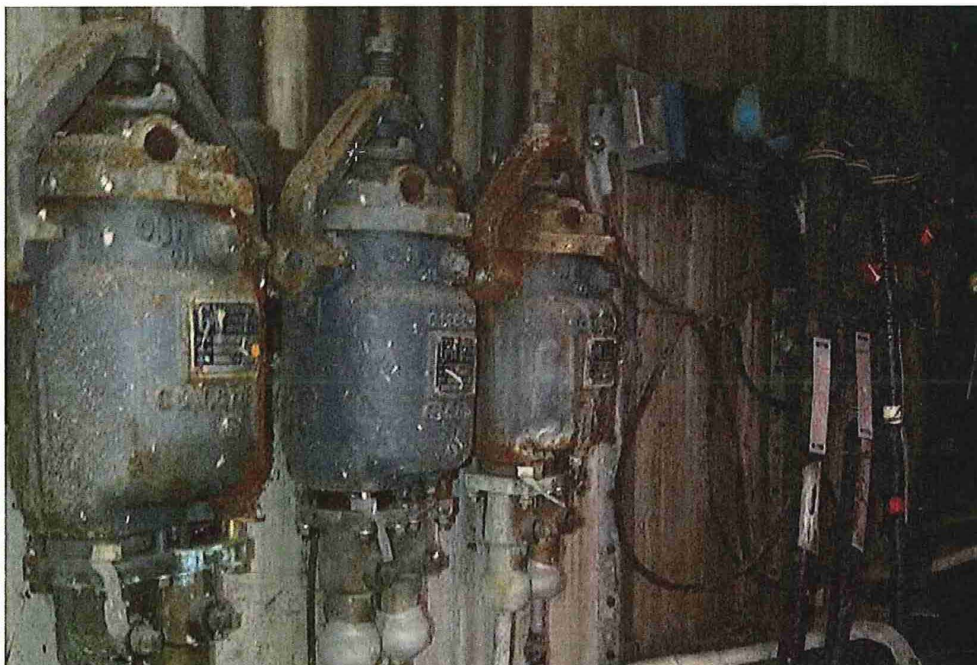
Figure 10 - Open loop vault 1, Oil fuse cutout and junction bar shown
