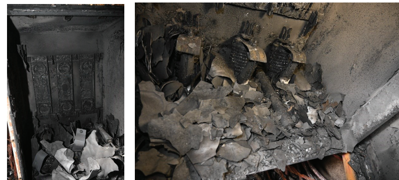
Figure 27: CLF cabinet inside (left); fuses and components found in debris at bottom (right).
