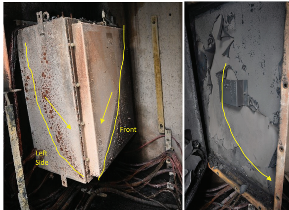
Figure 24: Front-left side of CLF (left); inside of cabinet door (right).
