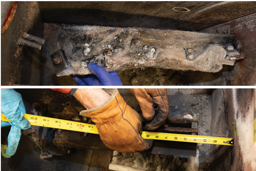
Figure 53: Service insulating board assembly showing gap at left side (top); supply insulating board from SW2018 positioned in SW2019 showing gap due to deformation of the SW2019 housing.
