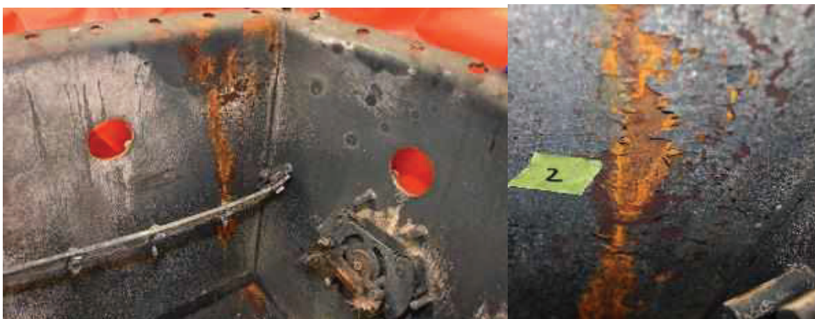
Figure 6. Close up photos of orange-brown areas inside of switch 2019 tank
