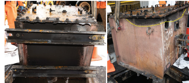
Figure 30: SW2018 back of housing - west side against the wall (left); left side and front (right).
