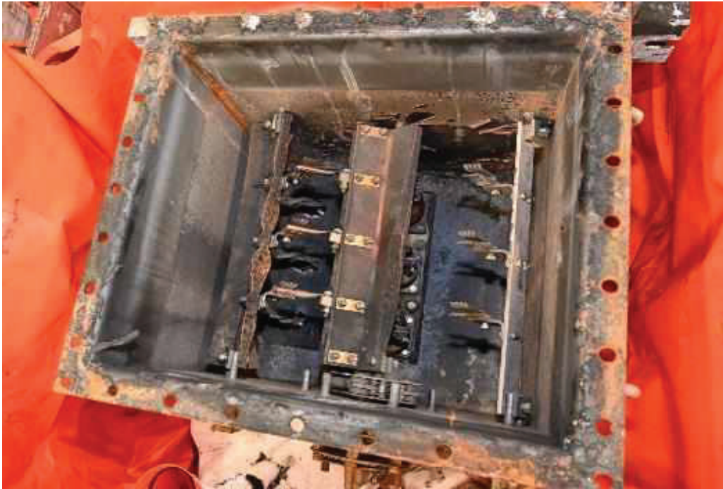
Figure 8. Top down view into switch 2018 (as received)
