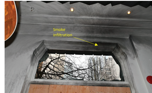
Figure 10: JJBean interior smoke extension dominant through south end of window.
