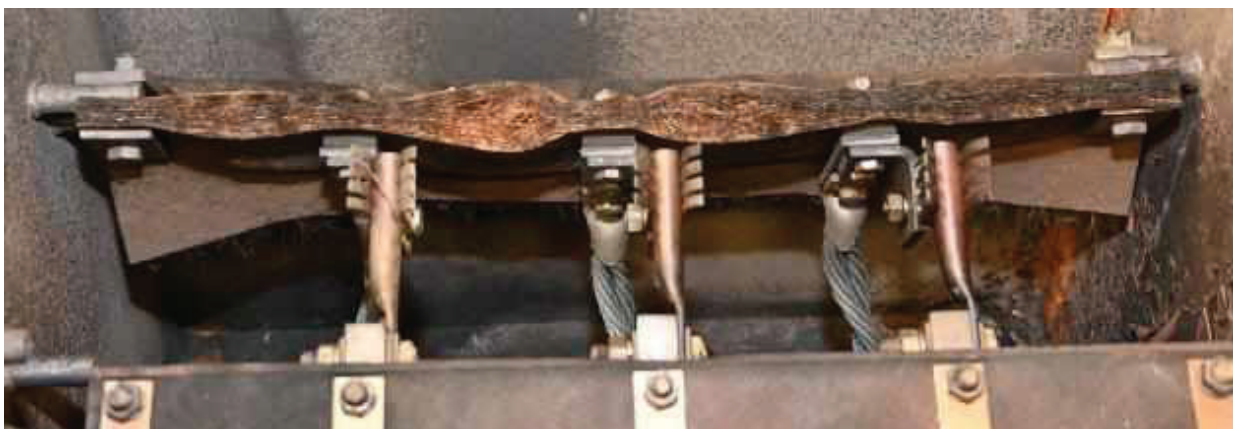
Figure 11. Insulating bar from switch 2018 showing expansion due to being exposed to high external heat
