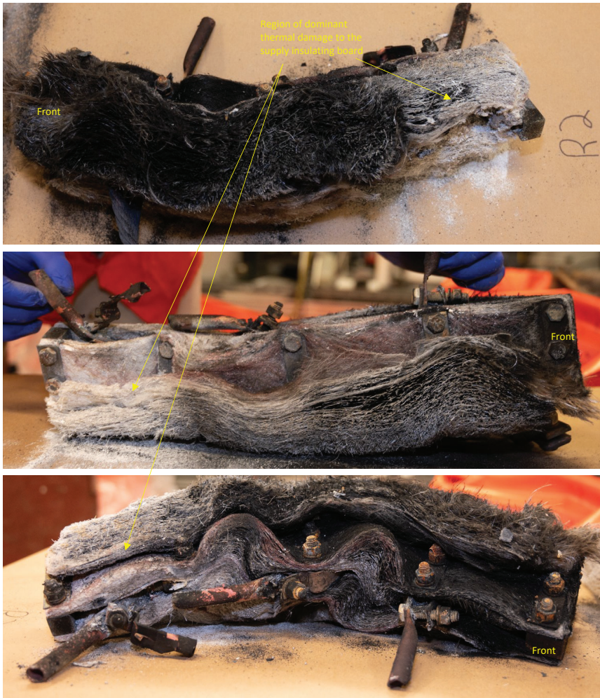
Figure 46: Images showing different views of supply insulating board with remaining blades and greater damage to the board at the back of the switch.
