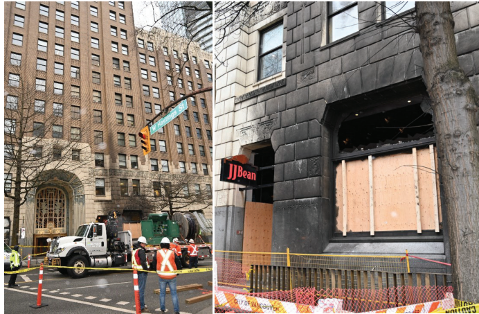
Figure 8: Marine Building façade damage.
