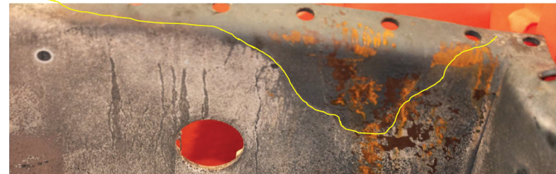
Figure 58: Region where no epoxy-enameled paint remained post-Incident.
