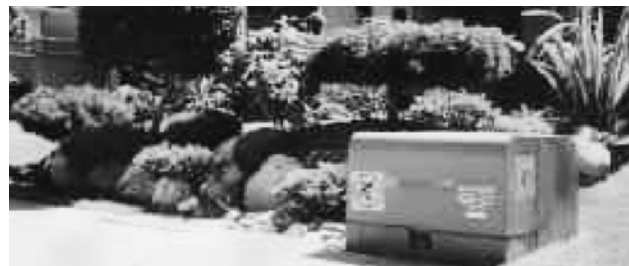
A good example of how plants and shrubs should be planted in the vicinity of a transformer unit.
