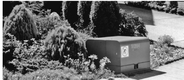
An example of plants and shrubs that have been planted too close to transformer unit.
