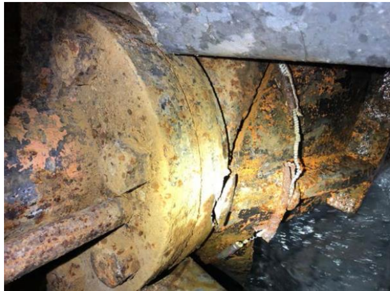
Figure 7 A large fracture was discovered in the body of Penstock Inlet Valve PIV01/02. This was the source of the leak and the uncontrolled flows down the penstock slope that created the Dam Safety Incident.
