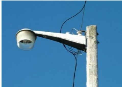
Figure 1: MV & HPS RS 1755 Outdoor Lights
