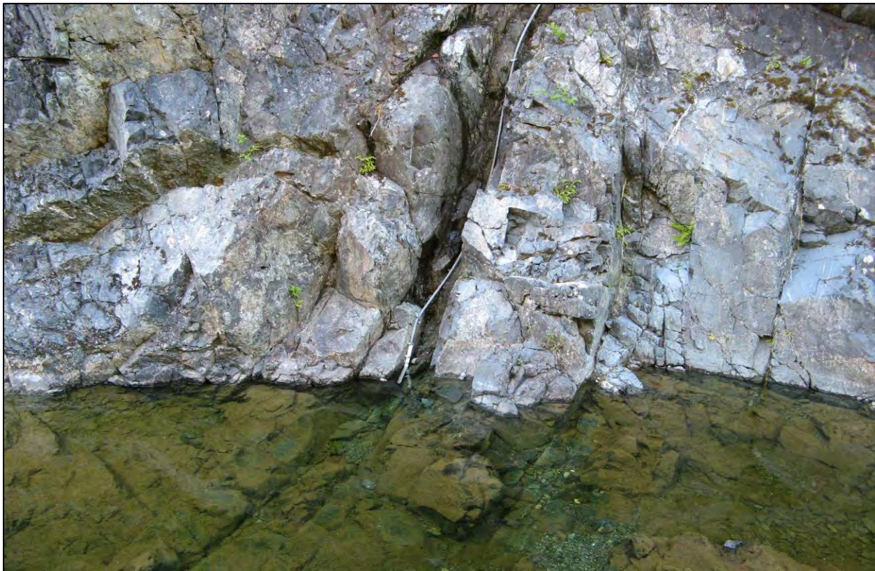
Photo 2. View of the transducer and cable installation at the M2 gauging station (2007–2011 location). The sensor was housed within a short section of PVC pipe while the sensor cable was encased in wire rope. Both were bolted to the bedrock wall at various locations.
