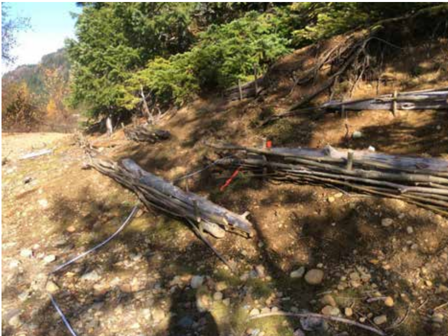
Figure 4. Slope stabilized with a combination of driftwood and wattle fences and stakes planted into terraces in D-3 treatment area at JHT-RV04 (plot JHT-PRM15) on October 28, 2019. Wattle fences are not woven around the stakes, but put on the up-hill side and backfilled with soil.
