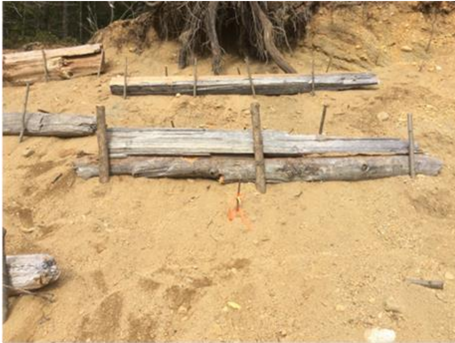
Figure 3. Slope stabilized with driftwood fences and stakes planted into terraces in D-1 treatment area at JHT-RV04 (plot JHT-PRM14) on November 6, 2019.
