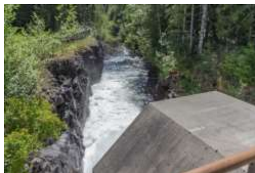
Photograph 1. Ash River Low Level Outlet. This outlet delivers pulse flows to the Ash River.
