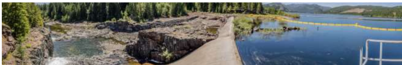
Photograph 3. Panorama of the Saddle Dam and Freecrest Overflow Spillway on Elsie Lake Reservoir.
