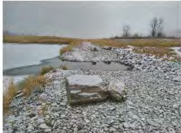
Photo 12: Looking south along former railway embankment at location of Site 15a outlet. Depth of water in outlet was 13 cm above invert. Note riprap proud of invert on left side of outlet.
