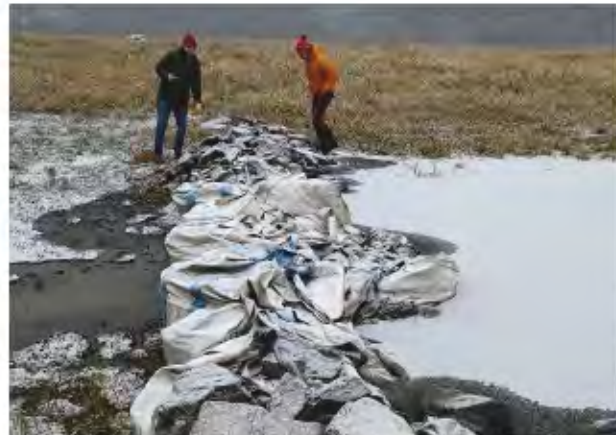
Photo 8: Looking west. Approximately 25 cm difference in hydraulic head between upstream and downstream of the bulk bag saddle dam.
