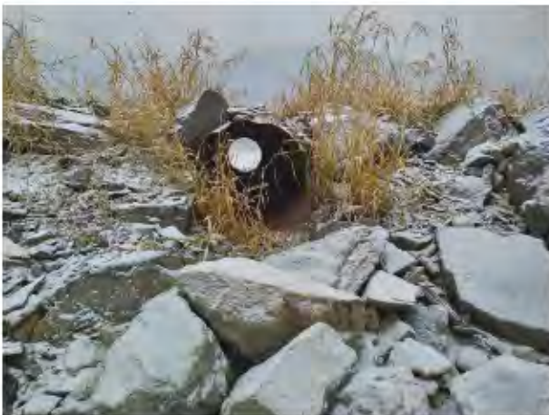
Photo 15: Looking east. 600 mm diameter CSP culvert approximately 10 m north of Site 15a outlet.
