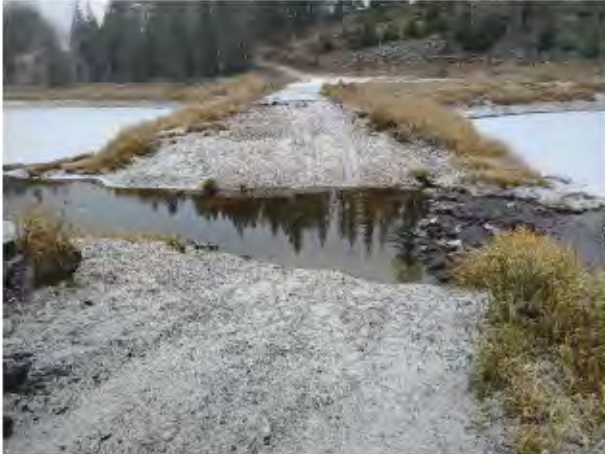
Photo 1: Looking south along alignment of decommissioned road separating upper and lower compartments of Cartier Bay. Water flow is from upper into lower compartment (left to right).
