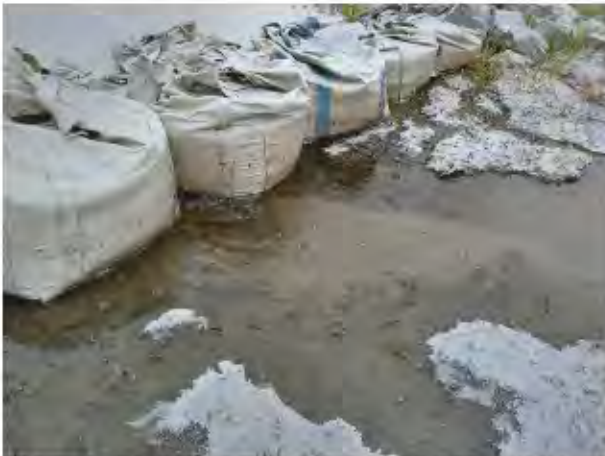
Photo 7: Downstream side of temporary bulk bag saddle dam above eroded channel at Area B. Sand and gravel spilled out of a torn bag and water was flowing between bags.
