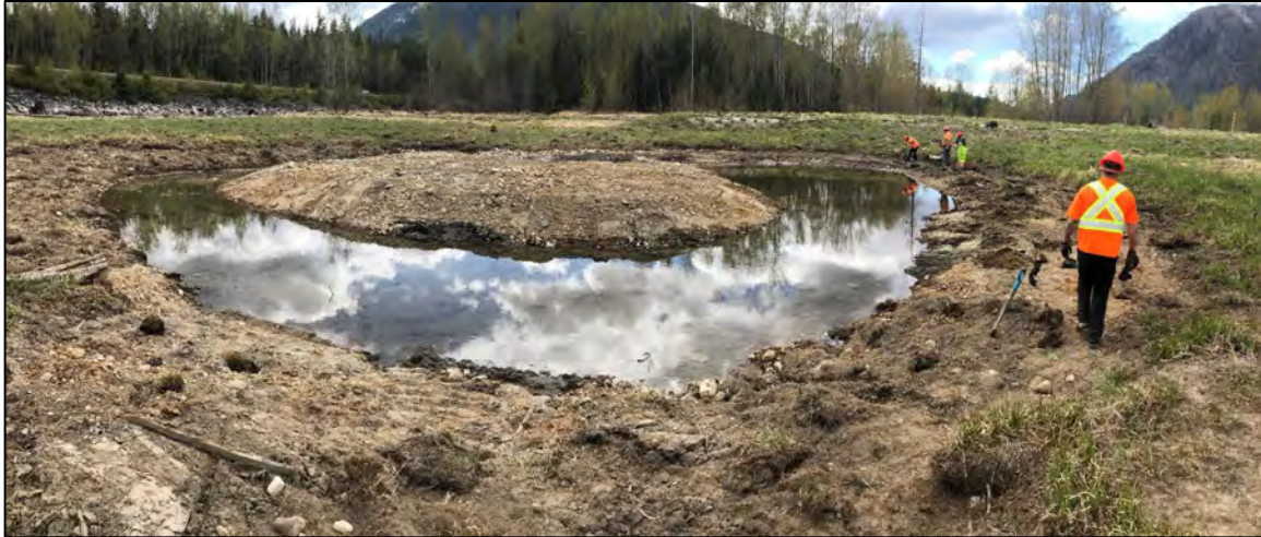
Figure 3-6. New (Phase 2) island feature, pond A2. Photographed in April 2021, shortly after construction, the island was planted in fall 2021 with nursery plugs of Kellogg’s and Columbia sedge. Photo: M. Miller.
