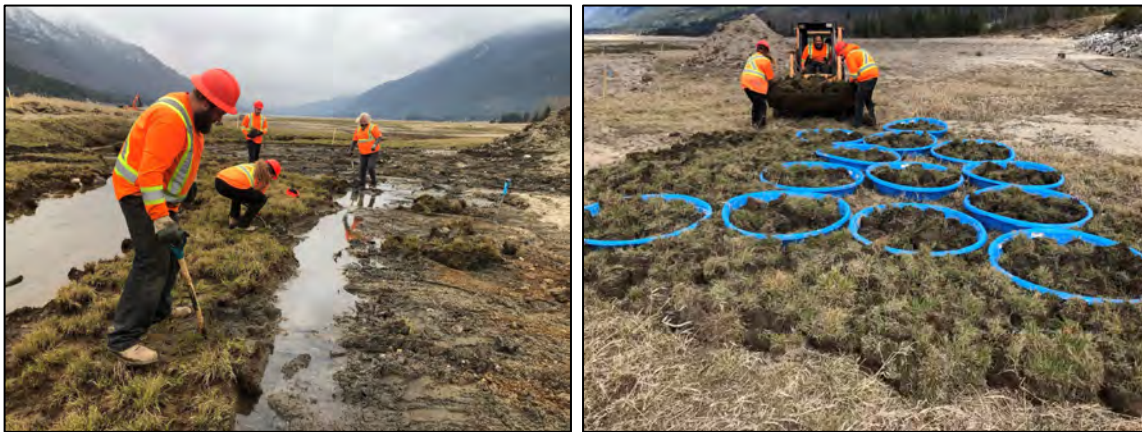
Figure 3-2. Native plant salvage. Left: stripping of sedge material from the footprint of pond A6. Right: off-loading salvaged plugs at stage area. Photos: M. Miller.
