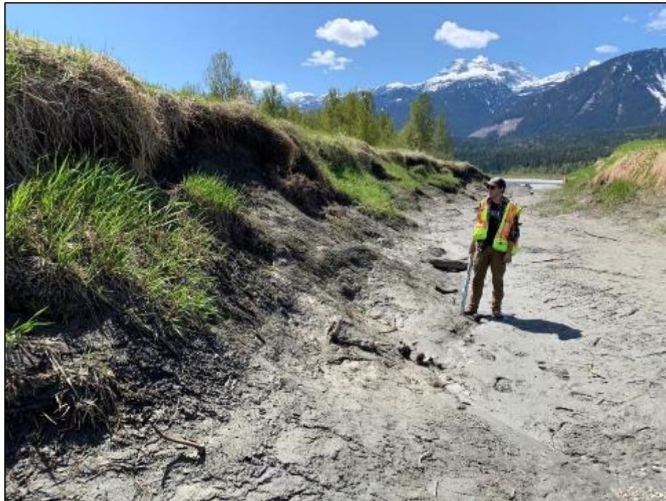
Figure 5-4: ONA field technician Addison Fosberry examining slumping and mass wasting in the main erosion channel at Site 6A. May 9, 2019.
