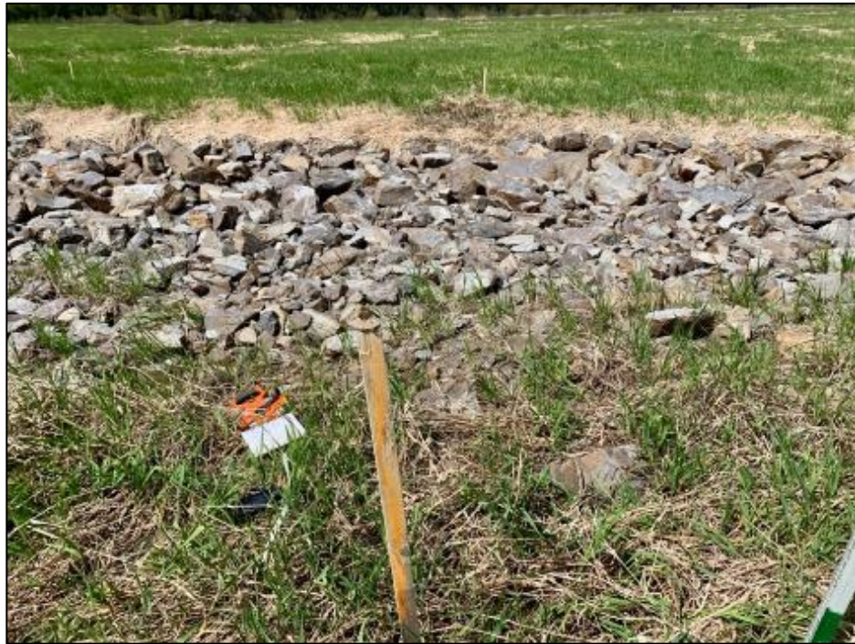
Figure 5-1: Reed canarygrass (in the foreground) ingressing into the riprap along the margin of the WPW-6A east erosion channel. Image Date May 9, 2019.
