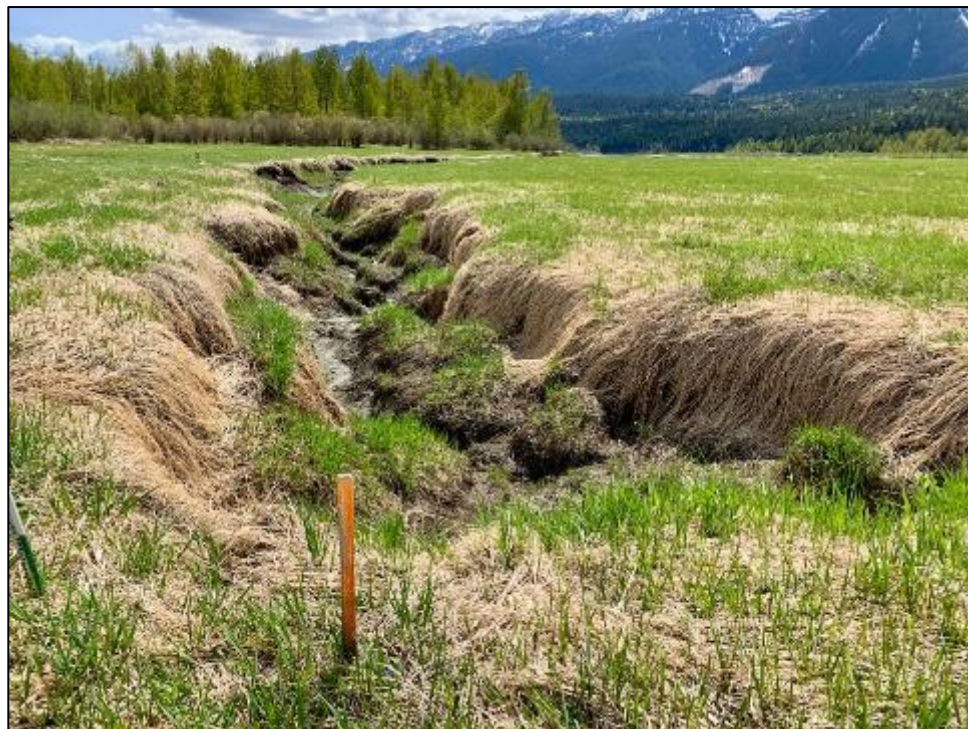
Figure 5-3: Extensive slumping and mass wasting in the WPW-6A west erosion channel. May 9, 2019.
