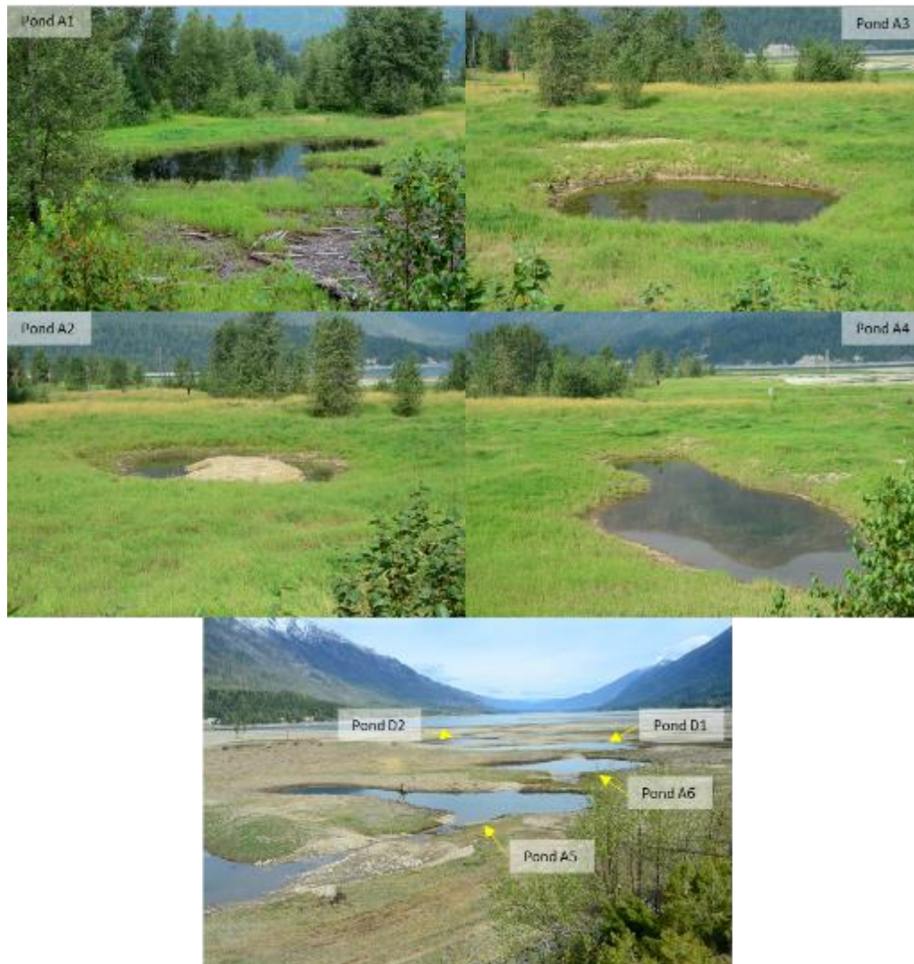
Figure 3-4. Photos of constructed ponds A1-A6, D1, and D2 taken at Burton Creek in 2021. Credit: G. Davidson. See Appendix A for a photographic time series (August to November 2021) of the constructed ponds A1-A4.
