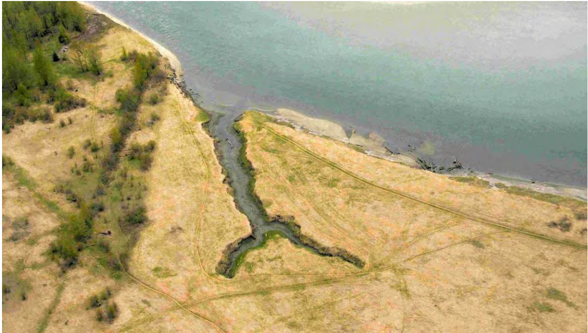
Figure 1-3: Collapsing erosion channel that will be fortified with a gravel blanket and rip-rap by WPW6A. Initially, the east branch will be treated as a trial to assess its effectiveness at preventing erosion
