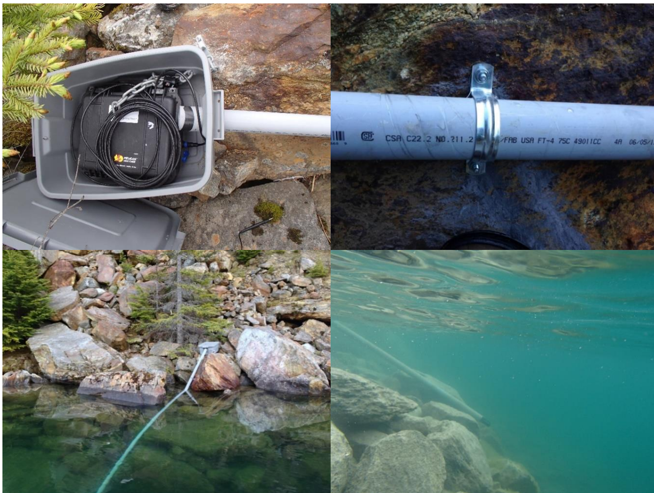
Figure 8-1. TGP monitoring station configuration including: a close up of the PT4 Pelican case anchored within a tote and the cable leading to the sonde through the standpipe (top left), a standpipe secured to a boulder with a hanger strap and expansion anchors (top right), an overview of Station 3 located 10.5 km from MGS (bottom left), and the submerged portion of a standpipe with the membrane protruding into the Columbia River (bottom right). Photos by: Evan Smith, Okanagan Nation Alliance (top left, bottom right) and Elmar Plate, LGL Limited (top right, bottom left).
