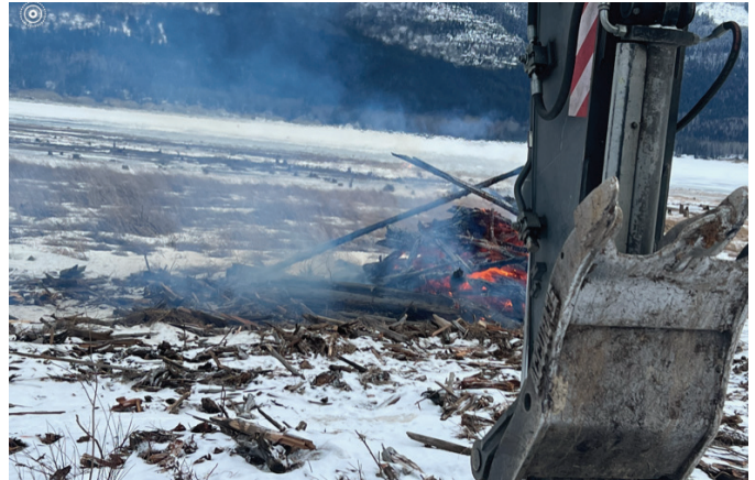
Excavator waits near burning debris pile in North Canoe Reach. Photo by Nathalie Dechka.
