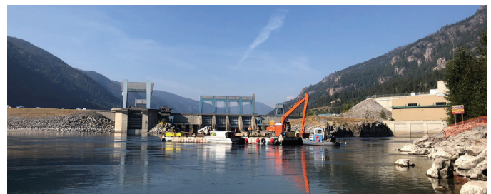
Enhancements were made to the sturgeon spawning site in the tailrace of Arrow Lakes Generating Station. Photo by Margo Sadler.
