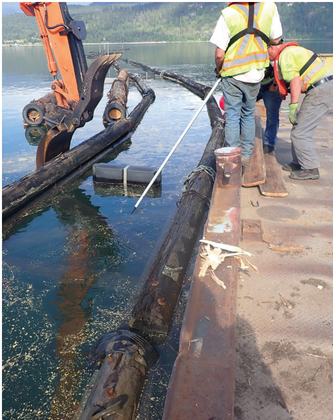
Repairs were completed on the Fauquier breakwater in the summer of 2022. Photo by Mical Dyck.
