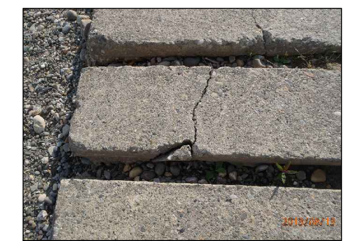
PHOTO No.2 TYP CRACKS TO PRECAST CONCRETE PLANKS AT EXISTING UPPER RAMP
