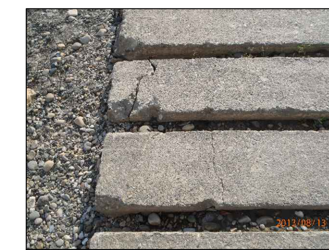
PHOTO No.1 TYP CRACKS TO PRECAST CONCRETE PLANKS AT EXISTING UPPER RAMP
