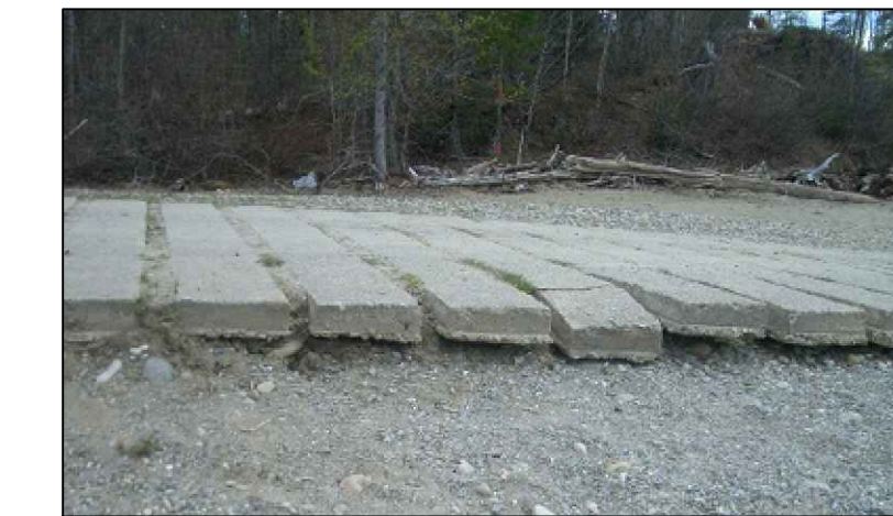
PHOTO No.3 SCOUR AND DAMAGE AT THE PRECAST CONCRETE PLANKS AT EXISTING UPPER RAMP. LENGTH & WIDTH OF UNDERMINED PLANKS TO BE FIELD MEASURED PRIOR TO SUBMITTING REMEDIATION PLAN.
