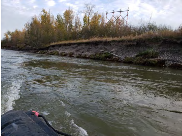
Photo 23 Peace River south bank erosion (north side of island) downstream of 102.5R
