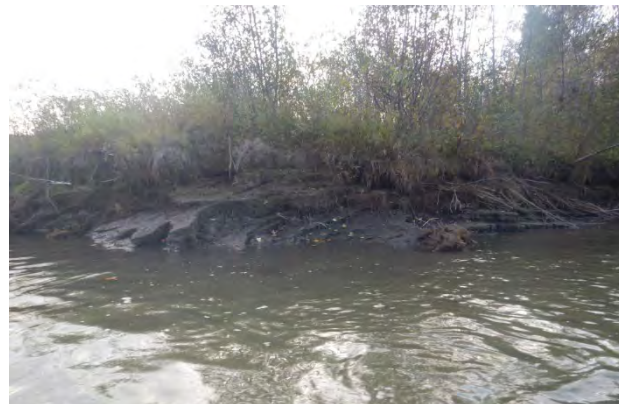
Photo 34 View of erosion of south bank of Peace River channel approximately 380 downstream from 102.5R
