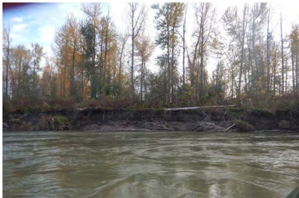
Photo 33 View of erosion of south bank of Peace River channel approximately 300 downstream from 102.5R
