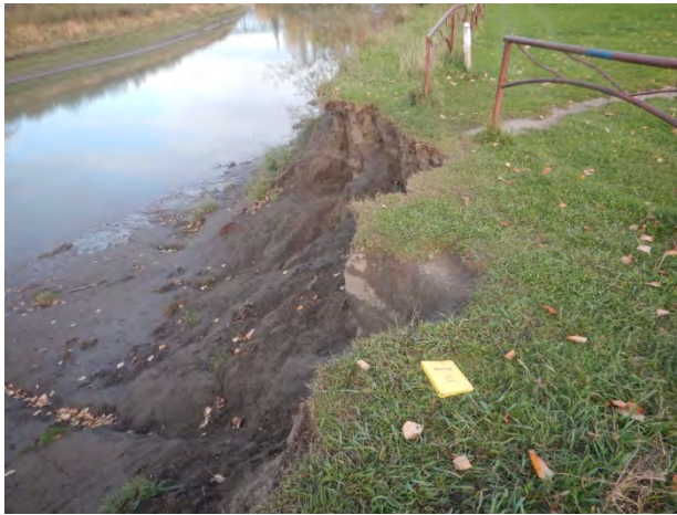
Photo 37 View east, Peace Island Park bank erosion
