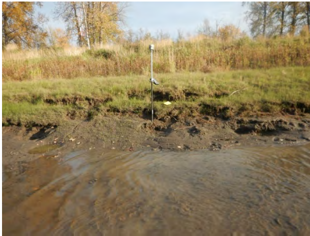
Photo 7 Section 4.5, left bank slumps
