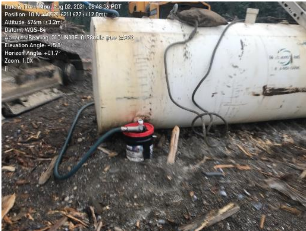
Figure 32: Fuel tank with drip containment at Peace Point
