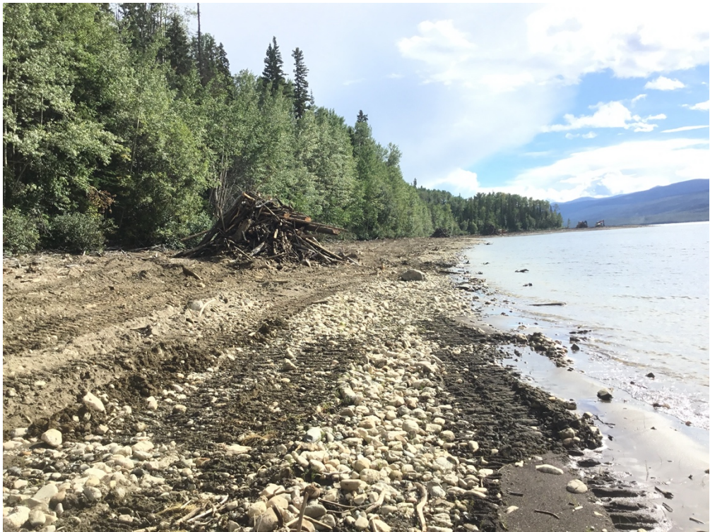
Figure 6: Davis North Beach after debris management, August 24,2020.
