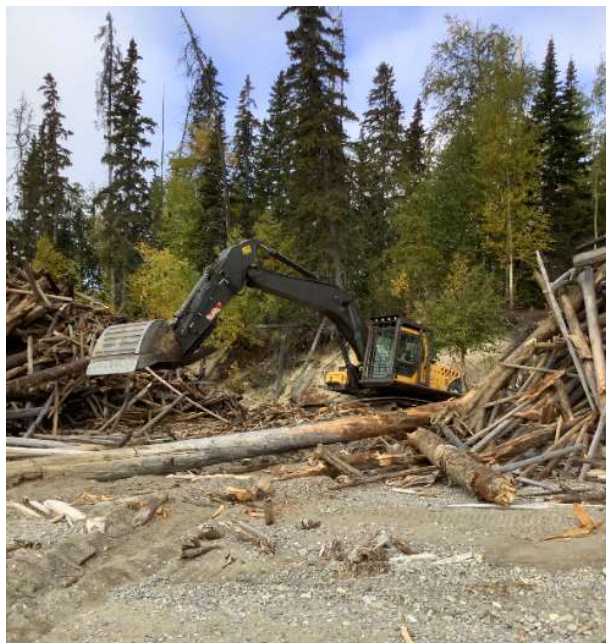
Figure 16: During Debris piling Factor Ross Beach
