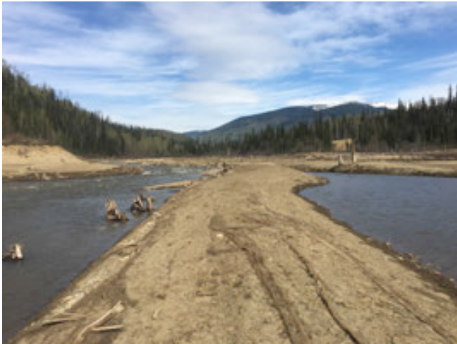
PHOTO 14: Berm 'F' Looking Upstream (Note Damaged/Decomposing ECM). Water on Right Side of Photo is Backwater from Reservoir, Not a Side Channel.
