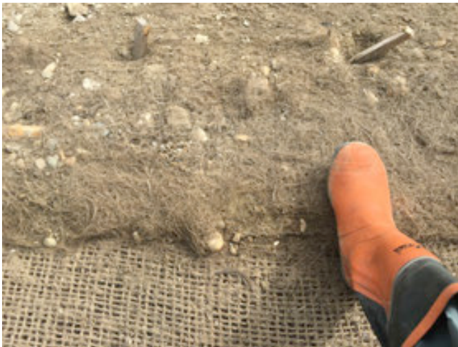
PHOTO 4: Deteriorating ECM (above) & Coir Soil Wraps in Good Condition (below)
