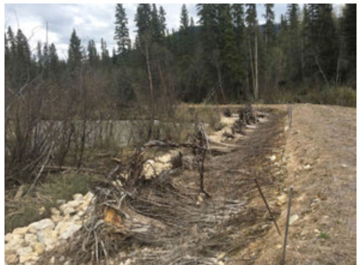
PHOTO 49: Coir soil wraps, willow brush layers, LWD, and riprap toe looking upstream
