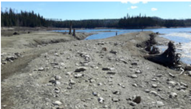
PHOTO 24: Material Used to Cover ECM When it Became Buoyant Still in Place.
