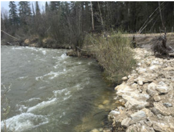
PHOTO 46: Eroding Bank and 'launching' riprap toe trench looking upstream
