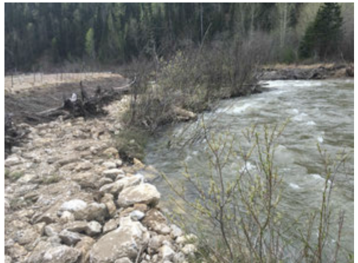
PHOTO 47: Eroding bank and 'launching' riprap toe trench looking downstream
