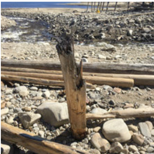
Photo 40: Broken upright log of the woody debris catcher
