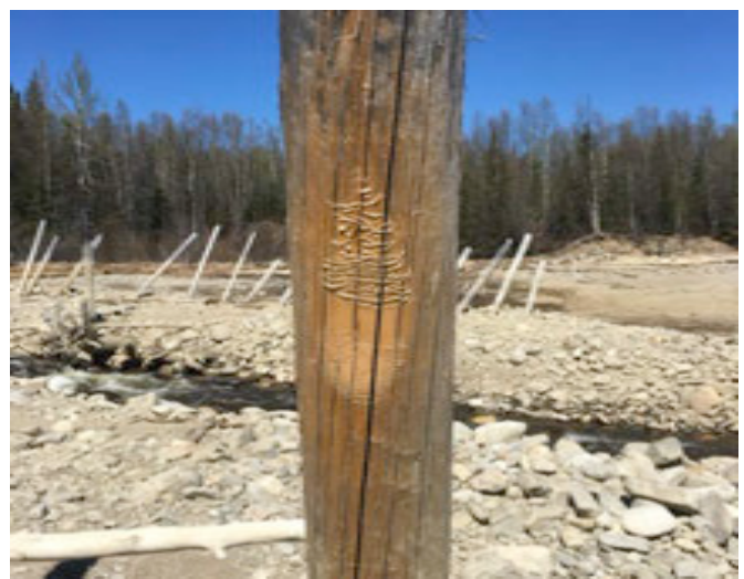
PHOTO 26: Damage to woody debris catcher
