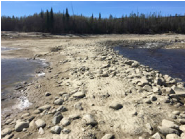
PHOTO 10: Looking upstream at Berm 'D' from downstream end of berm. Note erosion of fine fraction of the berm crest.
