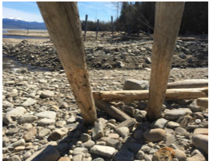
Photo 41: Damage to base of woody debris catcher upright logs
