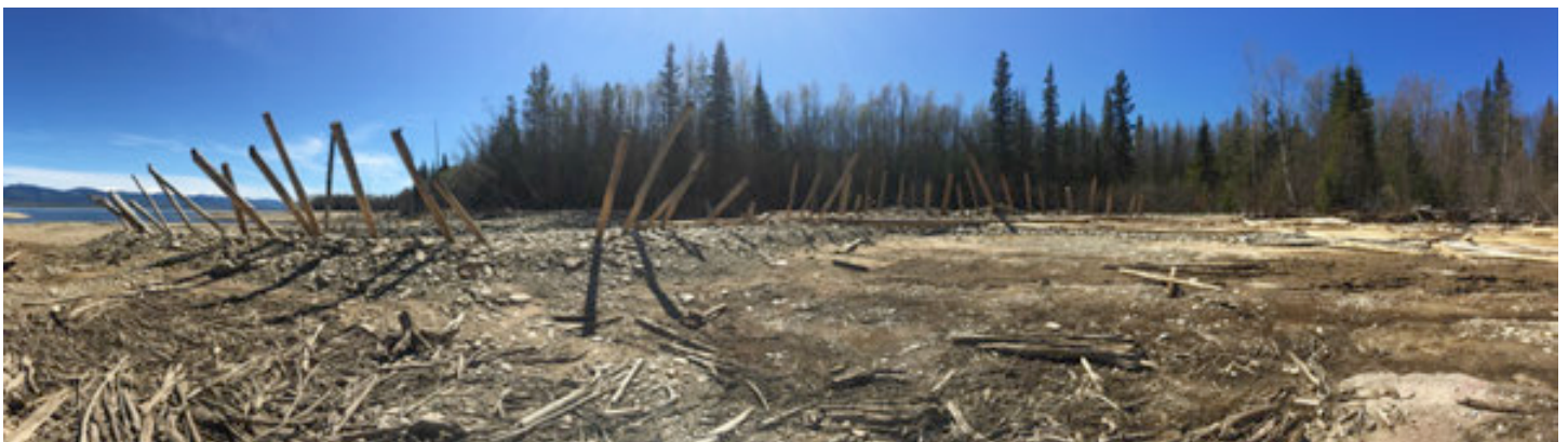
PHOTO 35 (Panoramic): Berm A and left bank woody debris catcher looking from left bank. Note some shifted and broken upright logs.
