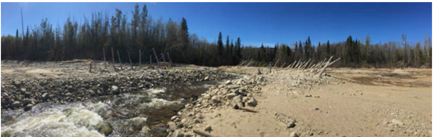
PHOTO 3 (Panoramic): Ole Creek works looking upstream at upper berms and debris catchers
