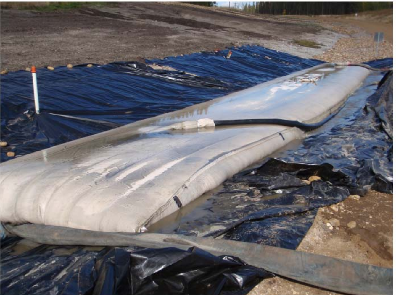
Photo 20: A geo-synthetic bag, similar to what would be used for WDS 34 Beaver Pond, being filled with dredged material.
