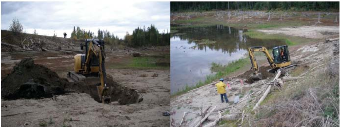
Photo 2: A mini-excavator was used to dig test pits at the base of the north side of the causeway.
