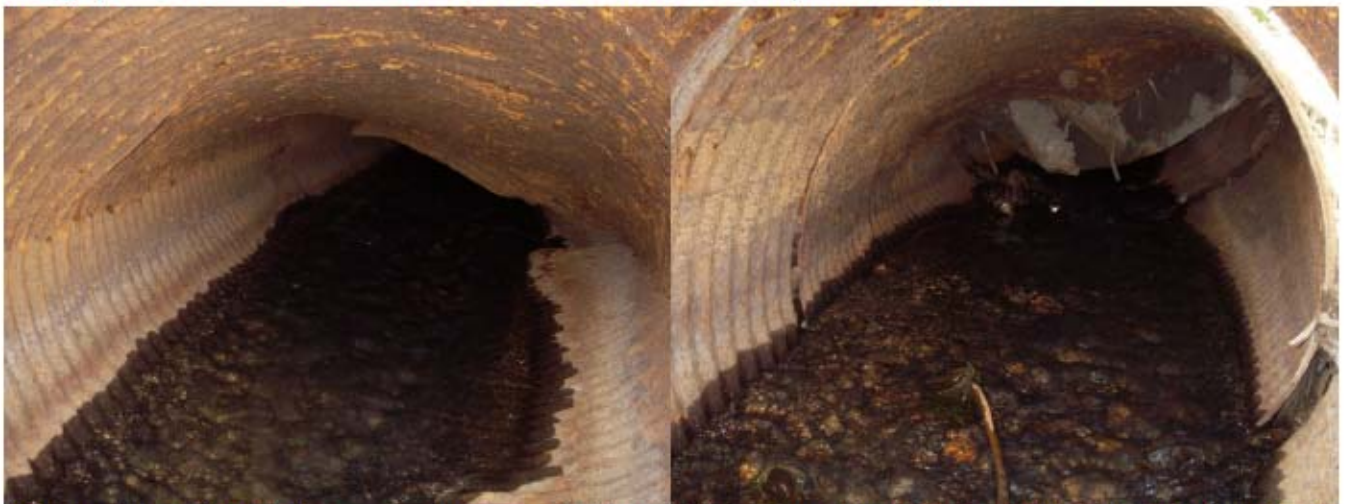
Photograph 9: Both culverts are showing signs of collapse. As is apparent from photosets 5 to 7, the existing culverts servicing the Airport Lagoon are in a state of disrepair, and are likely near the end of their service life.
