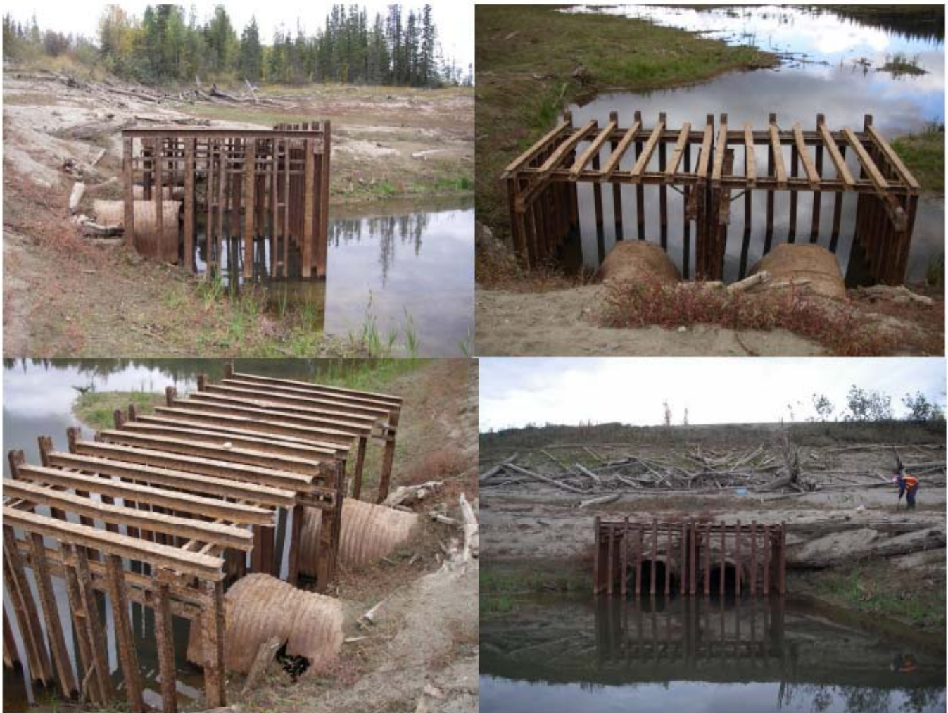
Photograph 11: Various views of the trash rack protecting the inlets of the 2 culverts on the north (upstream) side of the causeway.
