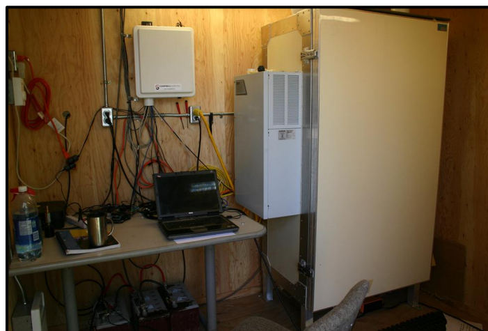
FIGURE 3.2. THE INTERIOR OF THE ENVIRONMENTAL ENCLOSURE SHOWING THE TEOM, DATALOGGING INSTRUMENTS, AND NETWORKING HARDWARE, TSAY KEH.
