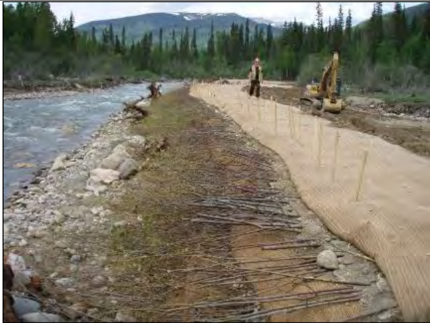
Photo C-2. Berm C – Downstream end of berm C with granular fill placed on the back side. Date taken: June 11, 2014.
