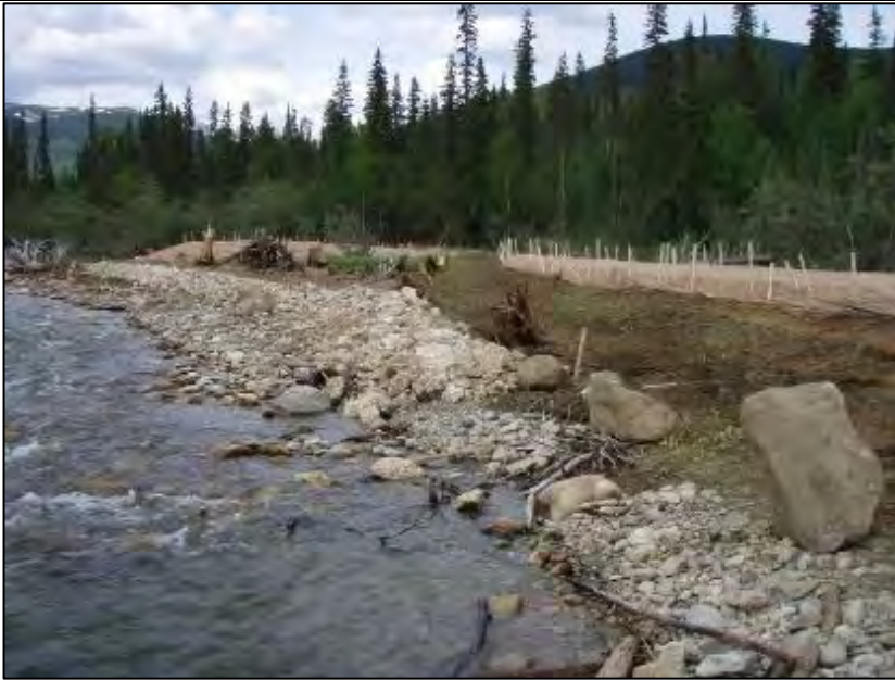
Photo C-1. Berm C – Upstream end of berm C and downstream end of berm J. Date taken: June 11, 2014.
