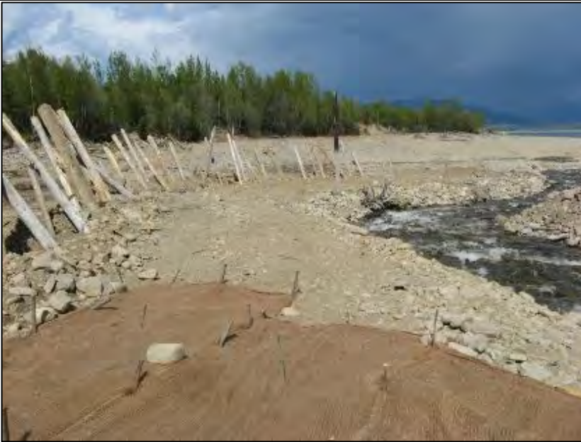
Photo A-1. Berm A – Downstream end of berm A, ECM use above EL. 671.0 m. Date taken: May 28, 2014.
