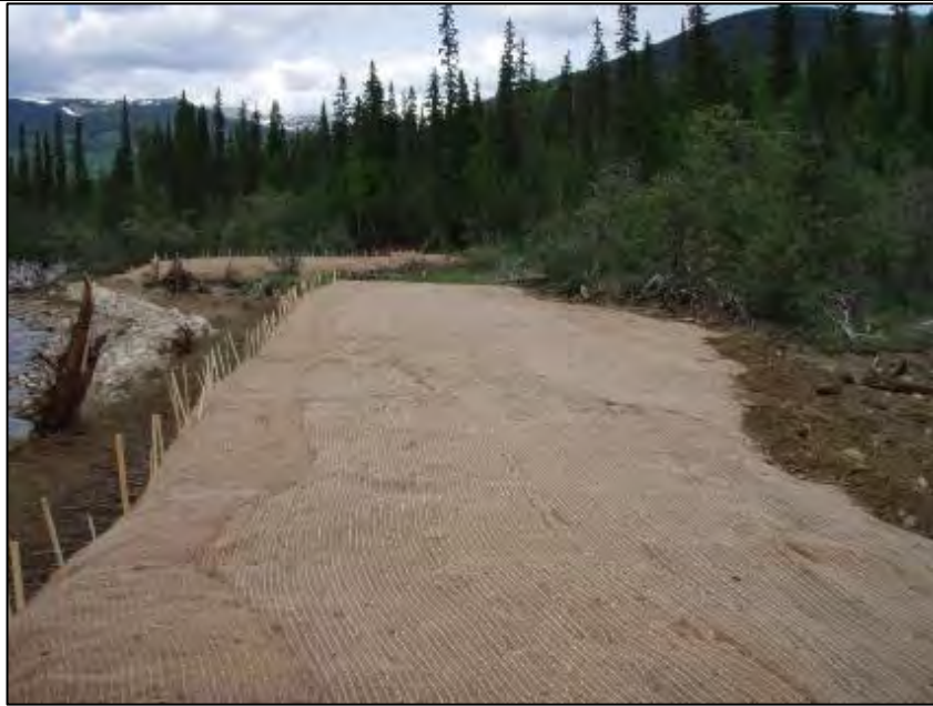
Photo C-3. Berm C – Upstream end of berm C and downstream end of berm J. Date taken: June 11, 2014.
