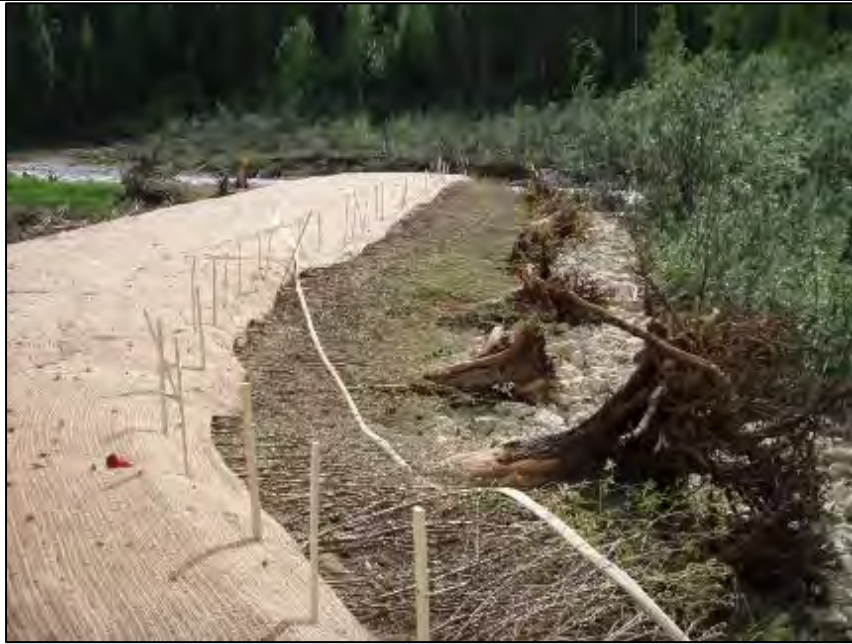
Photo J-2. Berm J – Midway along berm J looking downstream. Date taken: June 11, 2014.
