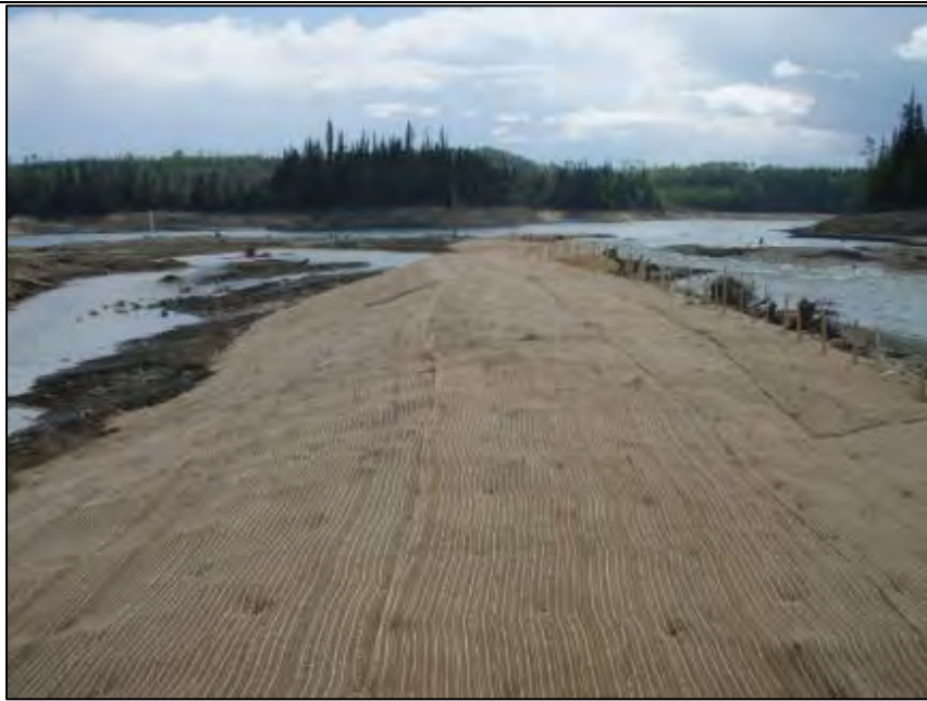
Photo DF-2. Berm D/F – Midway along berm F looking at berm G. Date taken: May 30, 2014.
