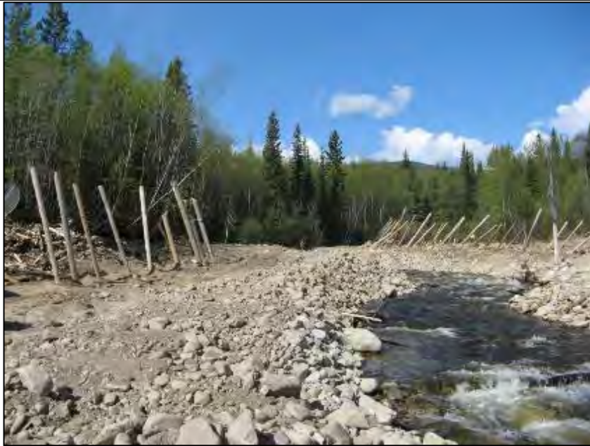
Photo C-1. Berm C – Upstream end of berm C with woody debris catcher. Date taken: May 28, 2014.
