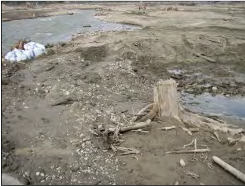
Photo A-2. Berm A – finished berm at ~0+900. The two front bulk bags to be removed. Date taken: May 20, 2014.
