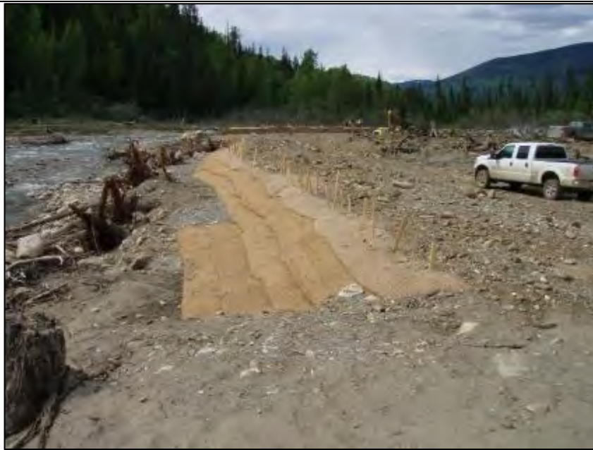
Photo B-3. Berm B – Downstream end of berm B, after ECM covered with granular fill. Date taken: June 11, 2014.
