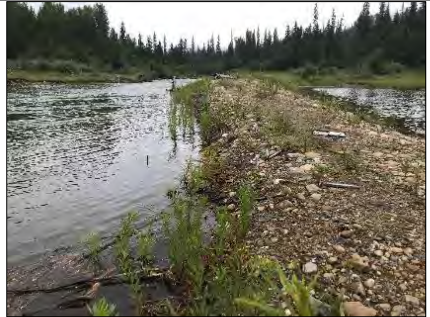
Photo C-2. Berm C – Downstream end of berm C with granular fill placed on the back side. Date taken: July 4, 2020.
