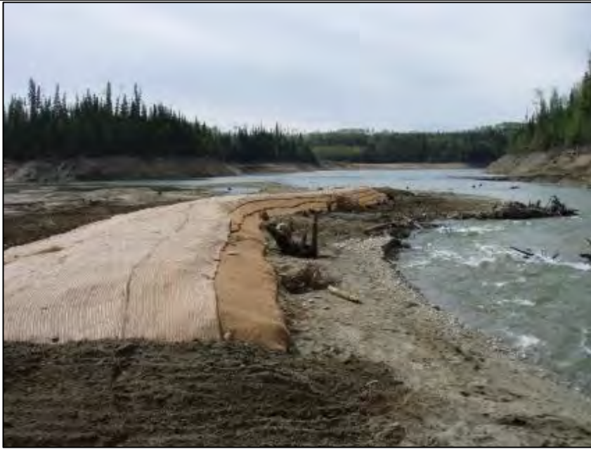
Photo G-1. Berm G – Upstream end of berm G, before all construction stakes were inserted. Date taken: May 26, 2014.
