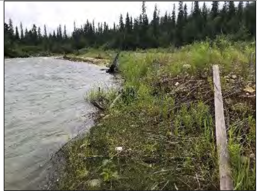
Photo C-1. Berm C – Upstream end of berm C and downstream end of berm J. Date taken: July 4, 2020.
