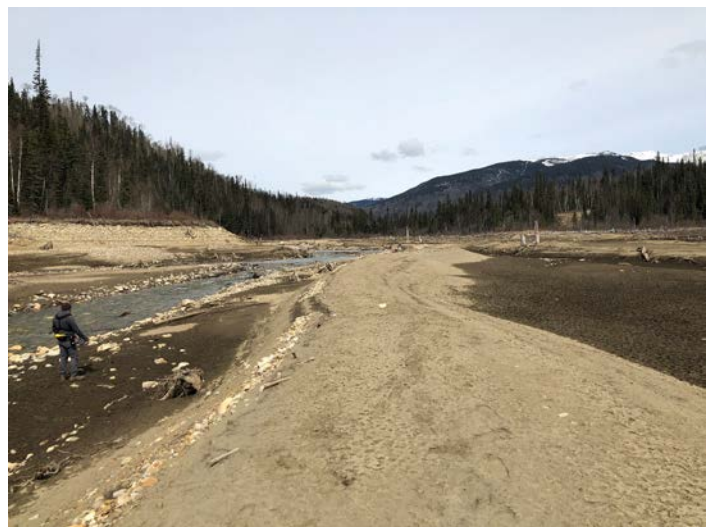
PHOTO 18: Berm 'F' Looking Upstream (Note Damaged/Decomposing ECM) (repeat of 2016 Ph#13)
