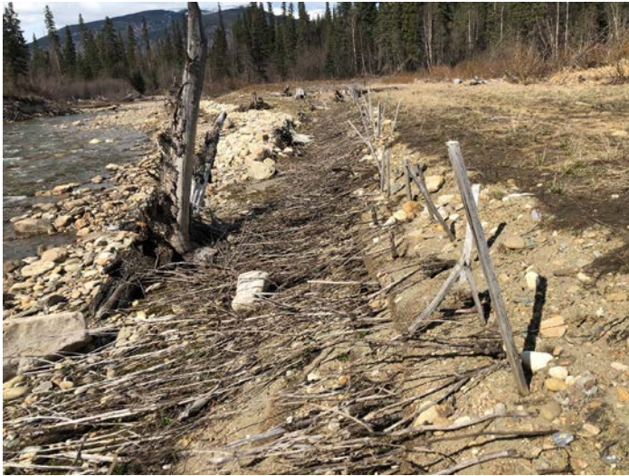
PHOTO 47: Few willow stakes took hold downstream berm area, but some growth (repeat of 2016 Ph#38)
