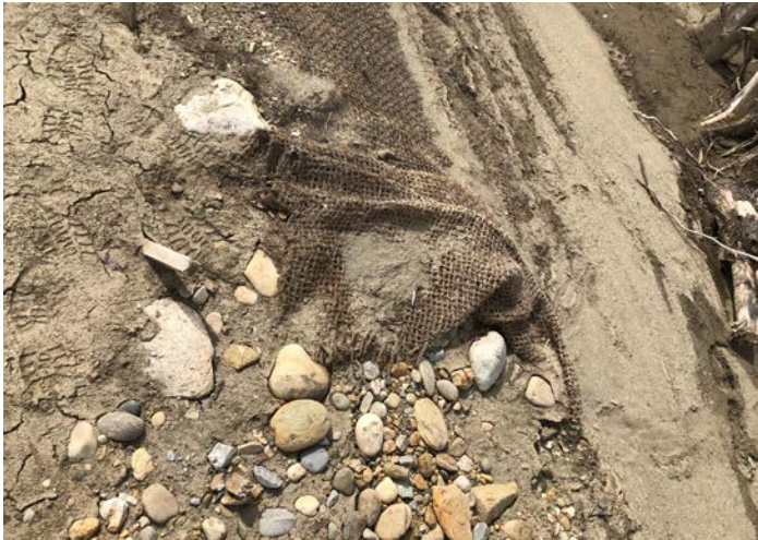
PHOTO 19: Coir Geogrid Matting becoming loose at the tie in between berm 'F' & 'D'
