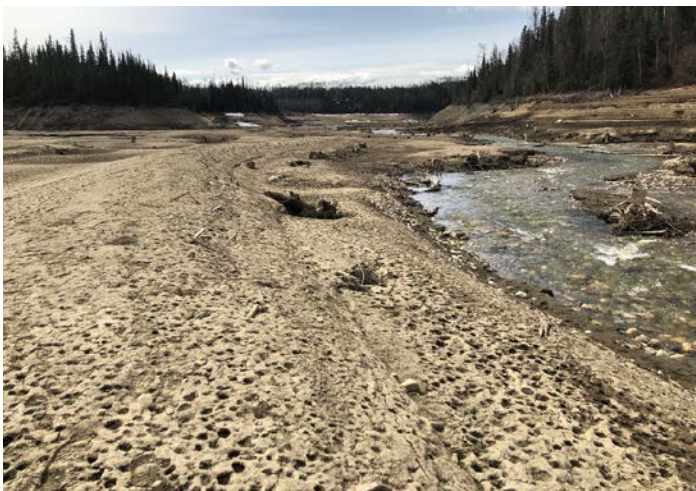
PHOTO 13: Survey of Toe of Berm 'G' on Creek Side (repeat of 2016 Ph#9)
