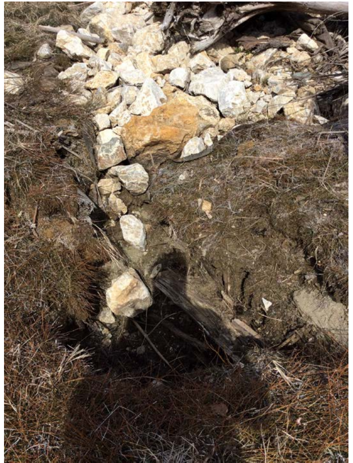
PHOTO 64: Erosion at downstream end of riprap toe protection
