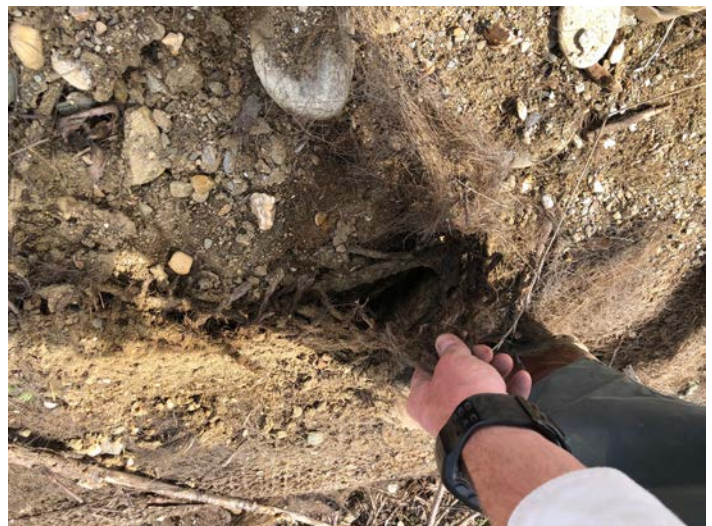
PHOTO 46: Damaged coir, perhaps due to ice or waves
