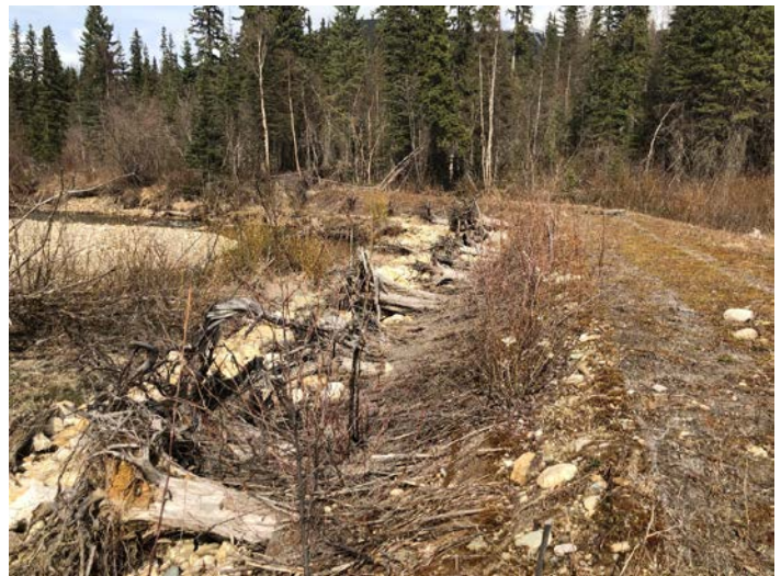
PHOTO 60: Coir Geogrid “Soil Wraps”, willow, LWD, and riprap toe looking upstream (repeat of 2016 Ph#49)
