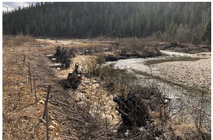
PHOTO 62: Soil wraps, willow brush layers, LWD and riprap looking downstream (repeat of 2016 Ph#51)
