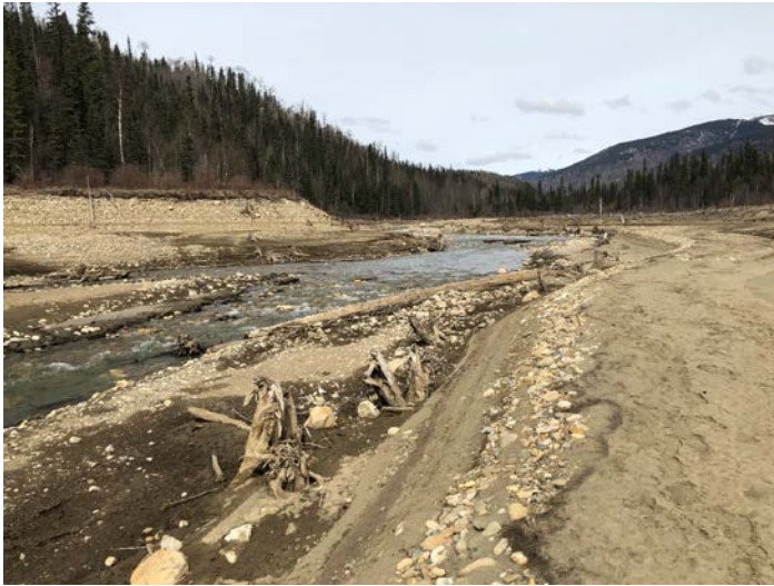
PHOTO 25: Deposited Log Along LWD and Deteriorating ECM (repeat of 2016 Ph#18)
