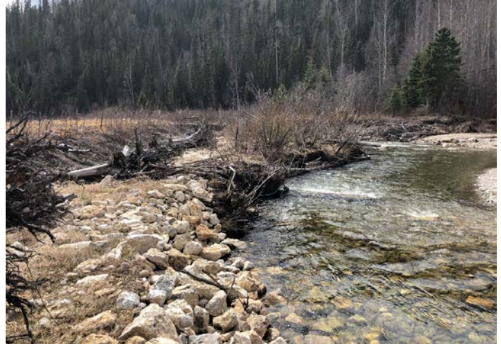
PHOTO 58: Eroding bank and ‘launching’ riprap toe trench looking downstream (repeat of 2016 Ph#47)
