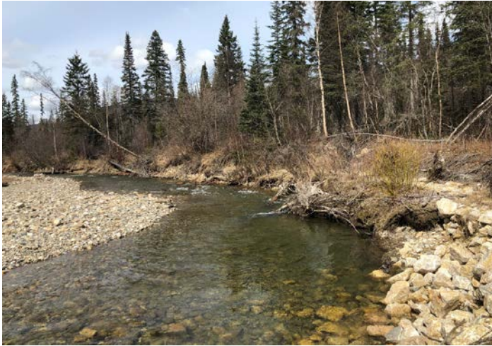
PHOTO 57: Eroding Bank and ‘launching’ riprap toe trench looking upstream (repeat of 2016 Ph#46)
