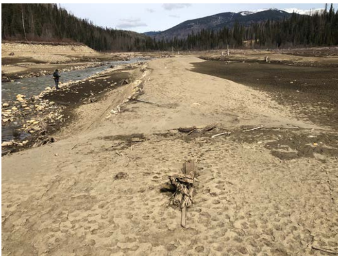
PHOTO 17: Downstream End of Berm 'F' Looking Upstream. Possible Erosion Downstream of Berm in 'Natural' Area (wet area in centre of Photo) (repeat of 2016 Ph#12)
