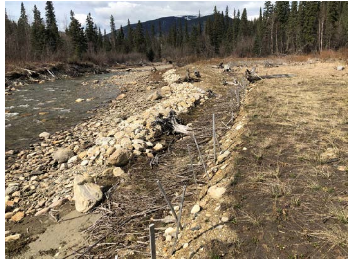
PHOTO 48: Looking upstream at willow layers in the lower berm and grasses on crest (no active growth given time of site visit) (repeat of 2016 Ph#39)
