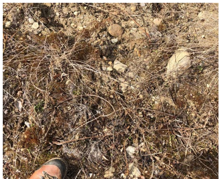
PHOTO 66: Moose related damage on back-side slope of berm (repeat of 2016 Ph#55)
