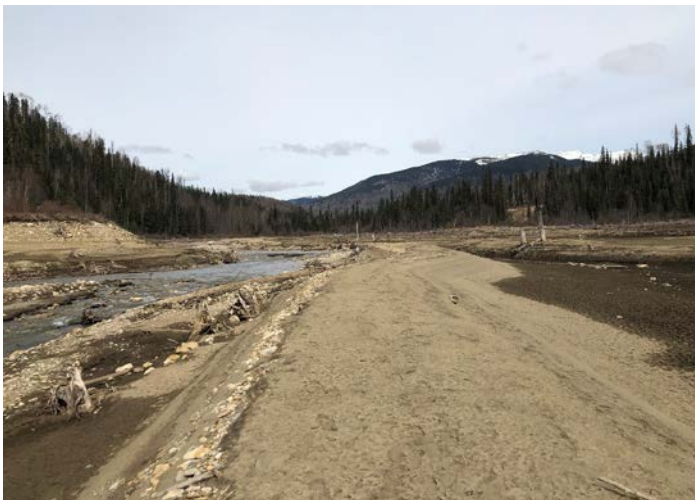
PHOTO 21: Berm 'F' Looking Upstream (Note Damaged/Decomposing ECM) (repeat of 2016 Ph#14)
