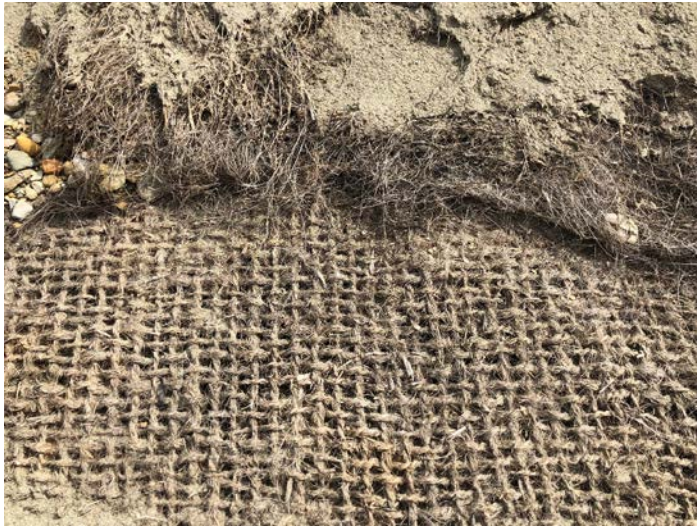
PHOTO 4: Deteriorating ECM (above) & Coir Soil Wraps in Good Condition (below) (repeat of 2016 Ph#4)
