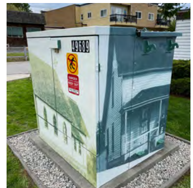
The Township of Langley added decorative wraps to BC Hydro equipment in their community
