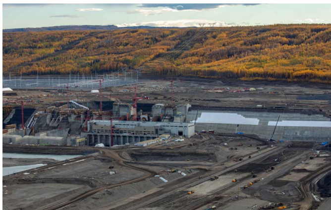
A view of the Site C dam core trench, dam buttress, powerhouse, spillways, and the operational substation in the background.
