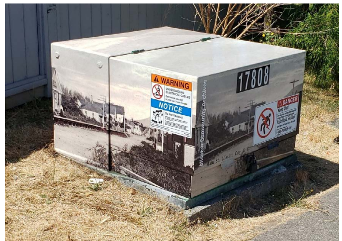
Example of a decorative wrap on our pad-mounted equipment in Mission.
