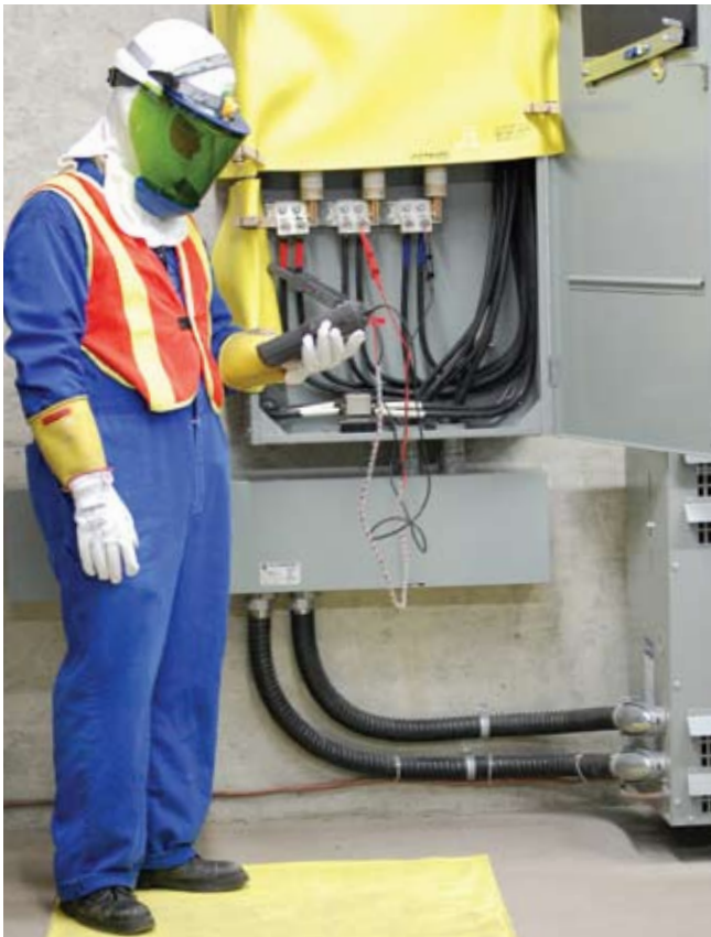
Measuring power factor on a branch circuit.
