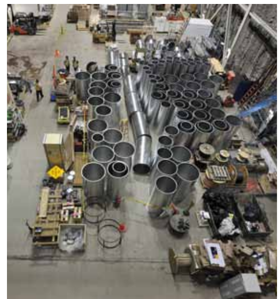
Tight space – storing equipment in Mica powerhouse.
