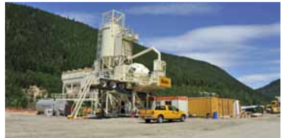
Mica batch plant that will produce concrete needed for installation of new generating units.
